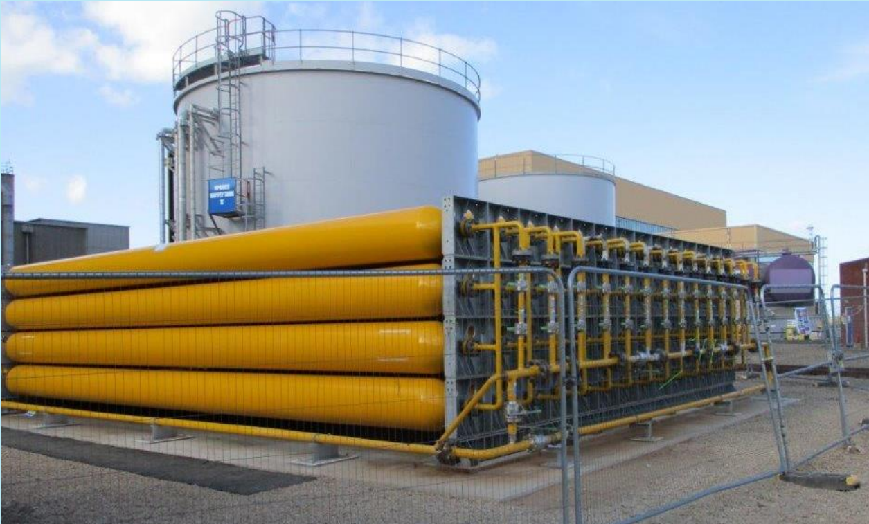
Figure 6.4: Secondary Shutdown System (Nitrogen Storage) at Hartlepool Power Station
