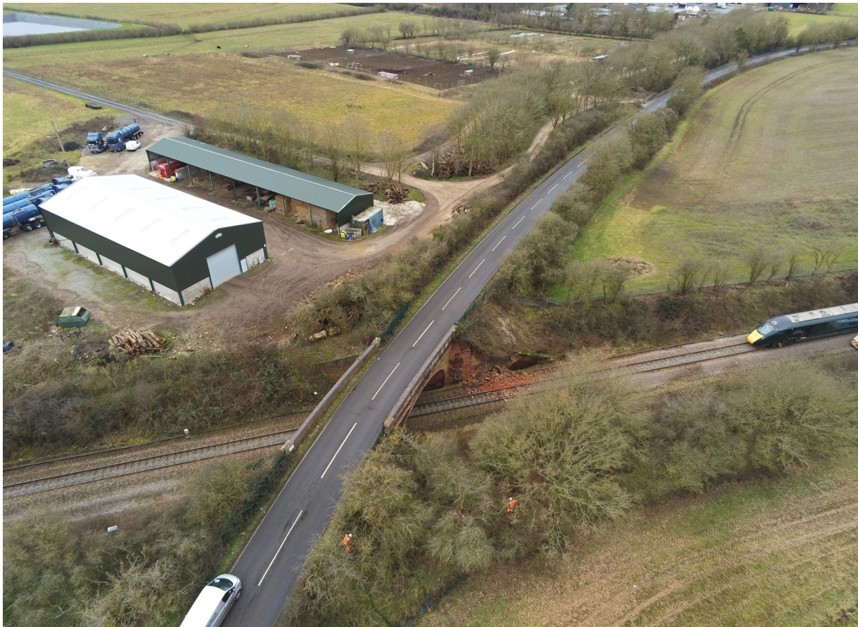
Figure 3: Overview on the morning after the accident showing the collapsed wing wall and rear vehicle of train 1W03 which stopped after passing under the bridge. The train was travelling from left to right.
