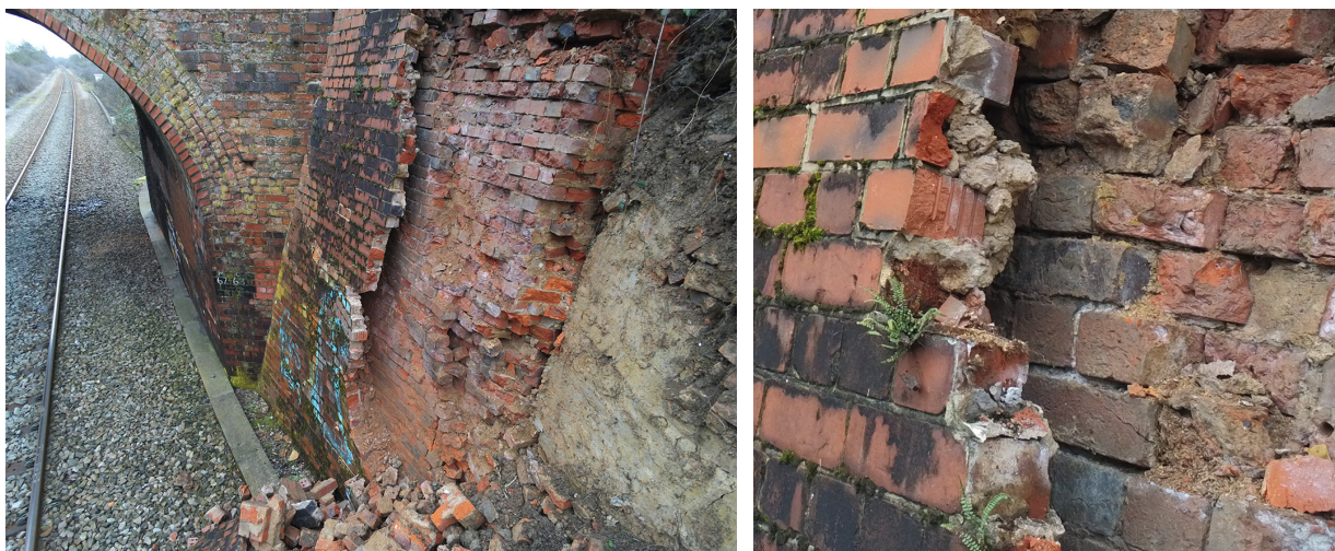
Figures 12a and 12b: View of partly collapsed wing wall and clay embankment core, and detailed view of skin wall showing short 'snap header' bricks and void around 100 mm wide.
