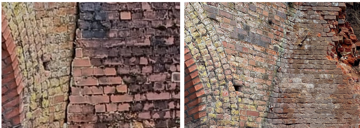
Figures 13a and 13b: Vertical fracture between skin wall and south abutment, and structural wall exposed after removal of skin wall (courtesy of Network Rail). Both images February 2023.
