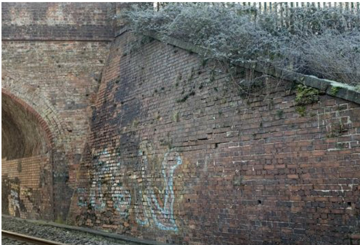
Figure 10: Image showing part of the south-west wing wall from the 2023 visual examination report captioned 'Appears to have increased bulging' (courtesy of XEIAD/Network Rail).
