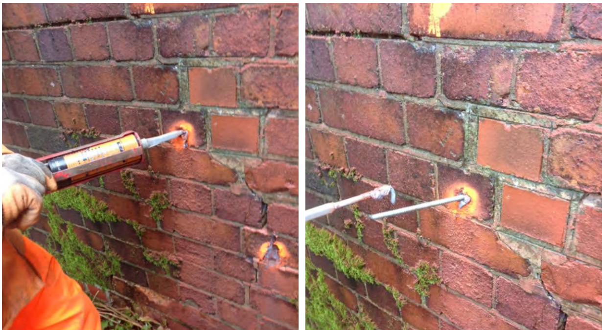
Figures 14a and 14b: Drill and grout repair in November 2013 (courtesy of QTS).
