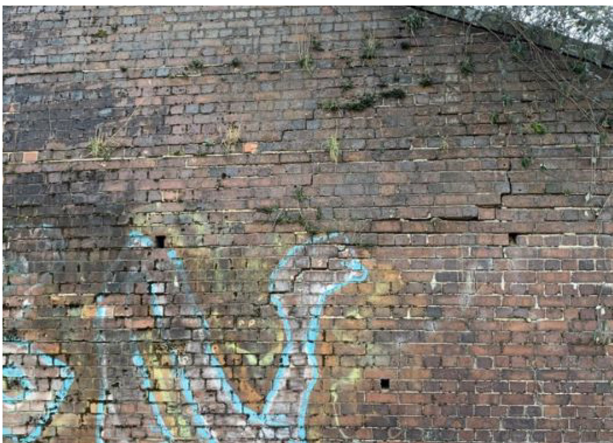
Figure 11: Image showing part of the south-west wing wall from the 2023 visual examination report captioned 'Deterioration throughout wall' (courtesy of XEIAD/Network Rail).
