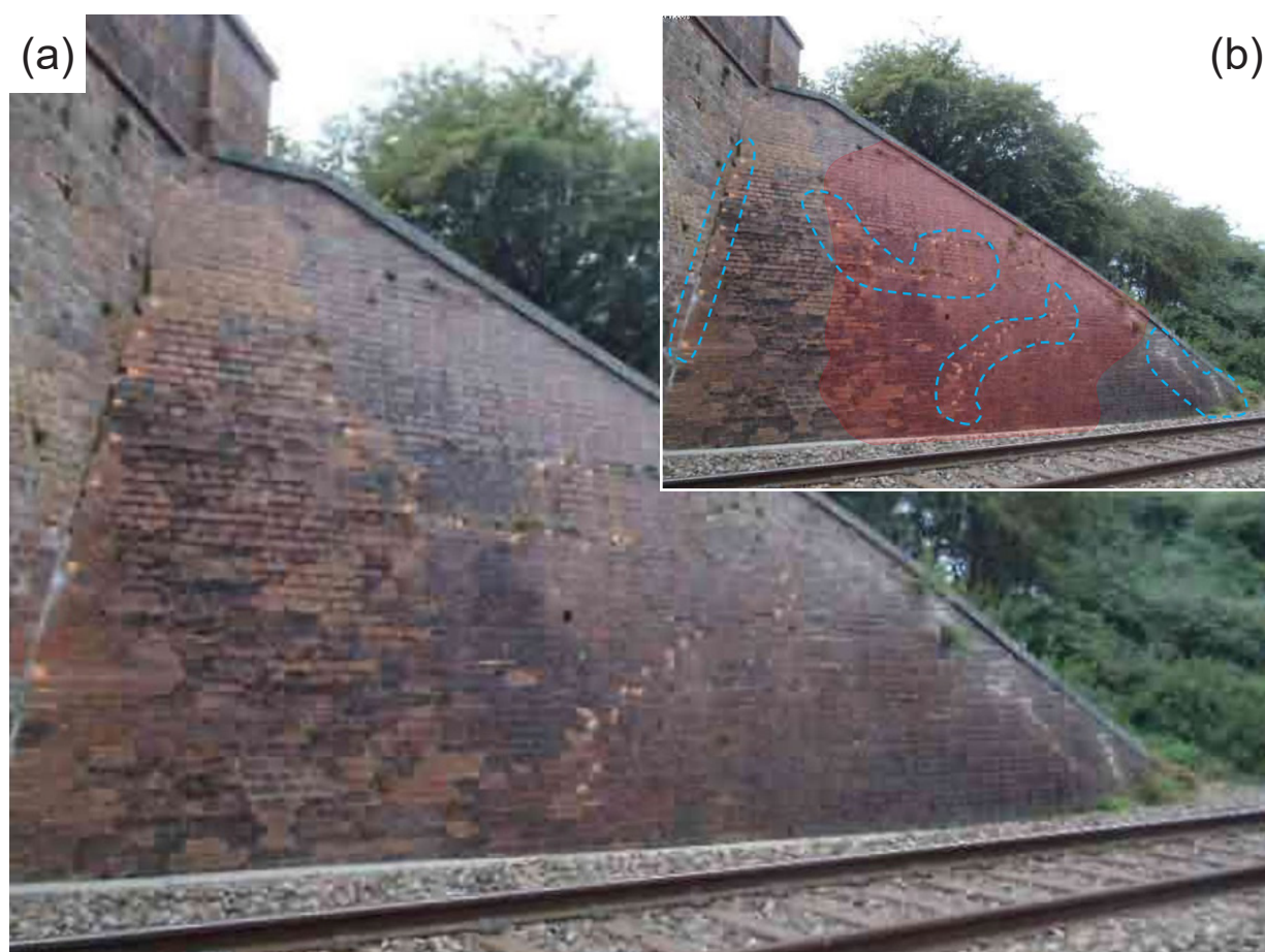
Figure 15: Image from the 2014 detailed examination report showing south-west wing wall and location of pin and grout repairs indicated by yellow paint marks (a), and with areas of repair outlined and area of collapse indicated by shading (b) (courtesy of Amey/Network Rail)
