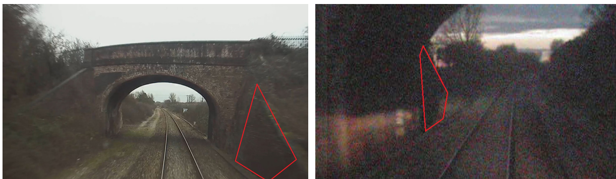
Figures 7a and 7b: Forward-facing CCTV images from passing trains at 16:29 hrs and 17:35 hrs. The section which later collapsed is outlined in red (courtesy of Great Western Railway).
