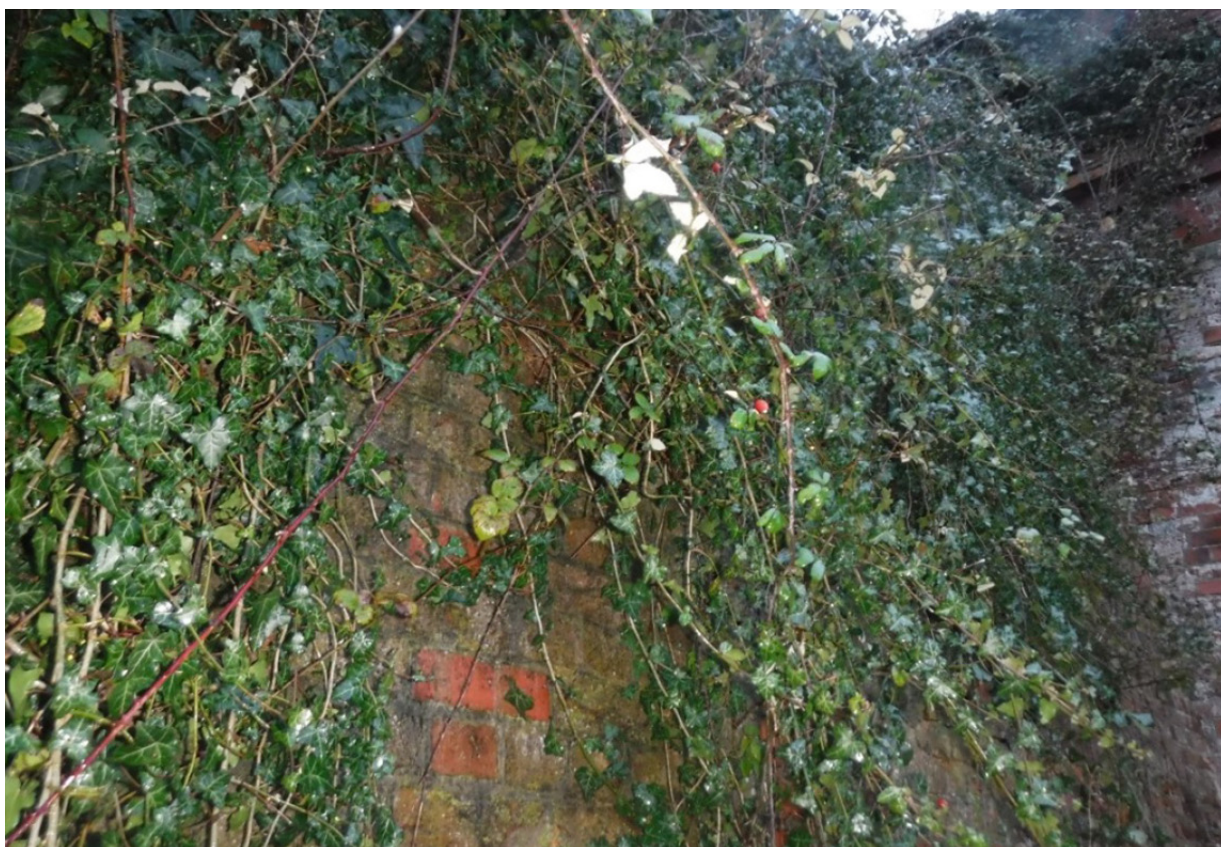
Figure 17: Image from 2021 detailed examination report showing vegetation growth obscuring the north-west wing wall (courtesy of Amey/Network Rail).
