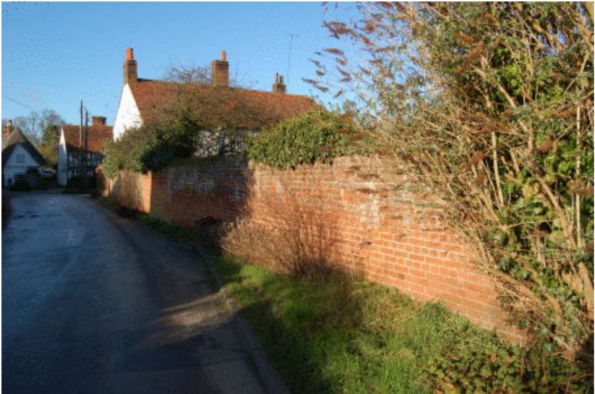
Picture 1.7 Quality boundary wall in English bond at the top of Middle Street
