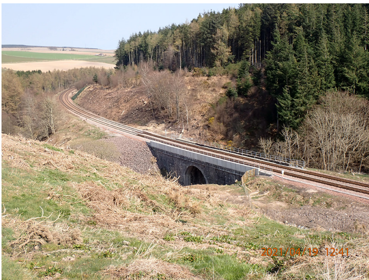
Figure F.9: Bridge 325 in April 2021 following the replacement of the down-side parapet and track
