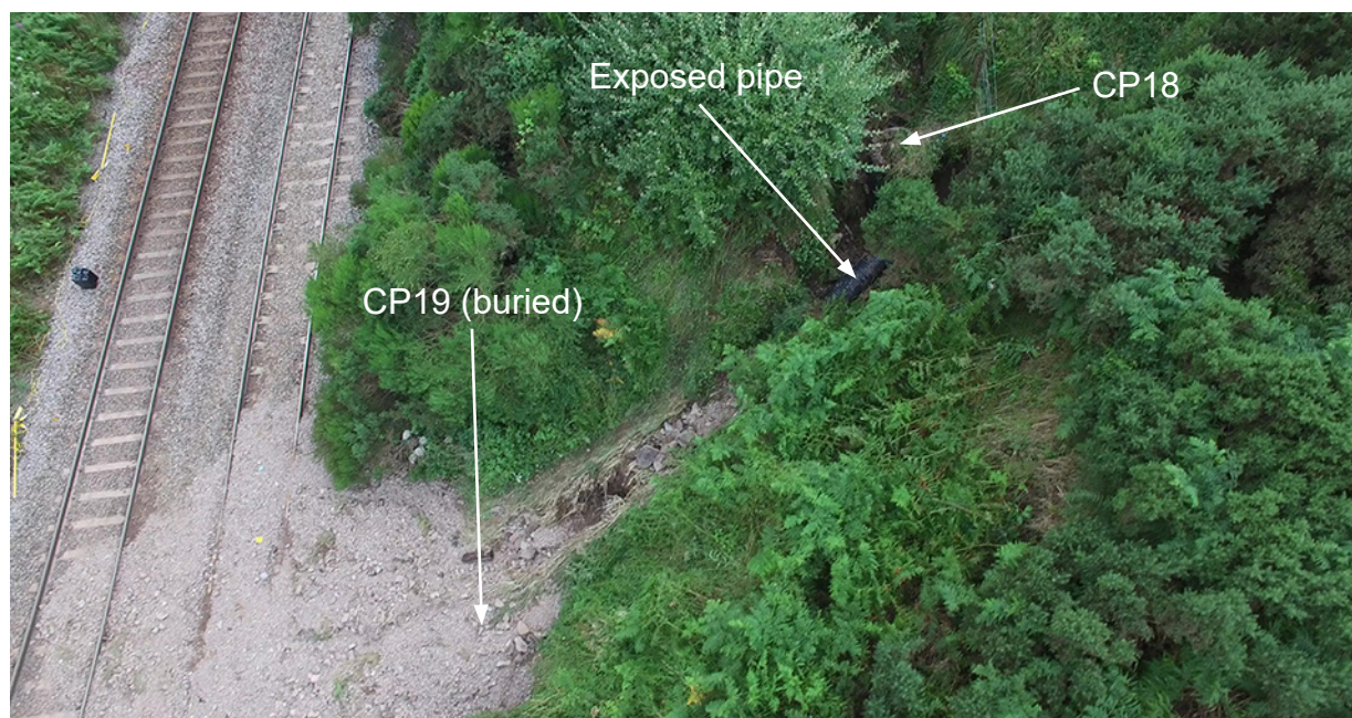
Figure 4: Washout debris on the track
