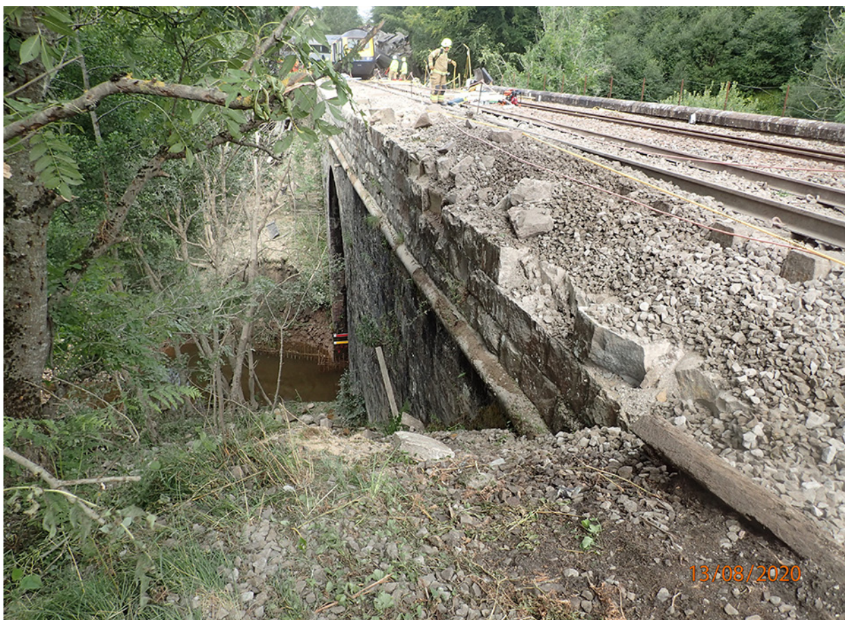
Figure F.5: Down-side parapet looking north showing damage to the parapet end
