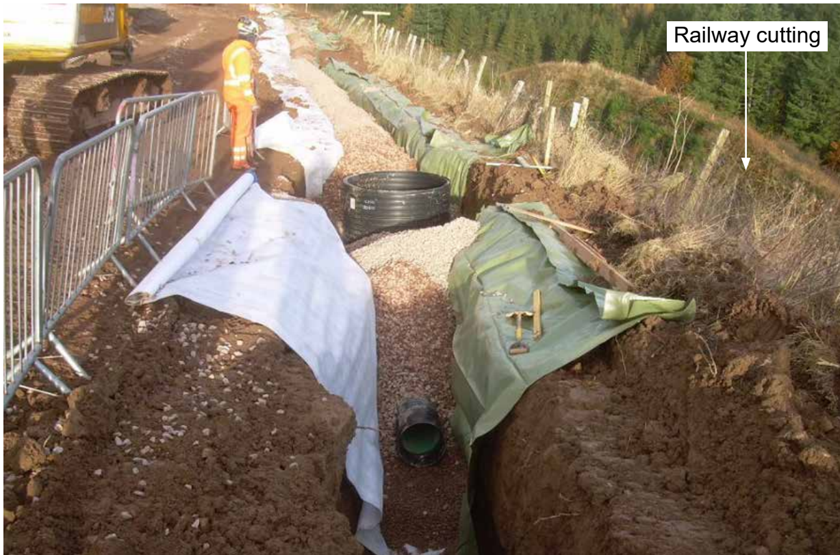
Figure 50: Drain under construction in late 2012 showing section between CP11 and CP16 looking north (Network Rail)
