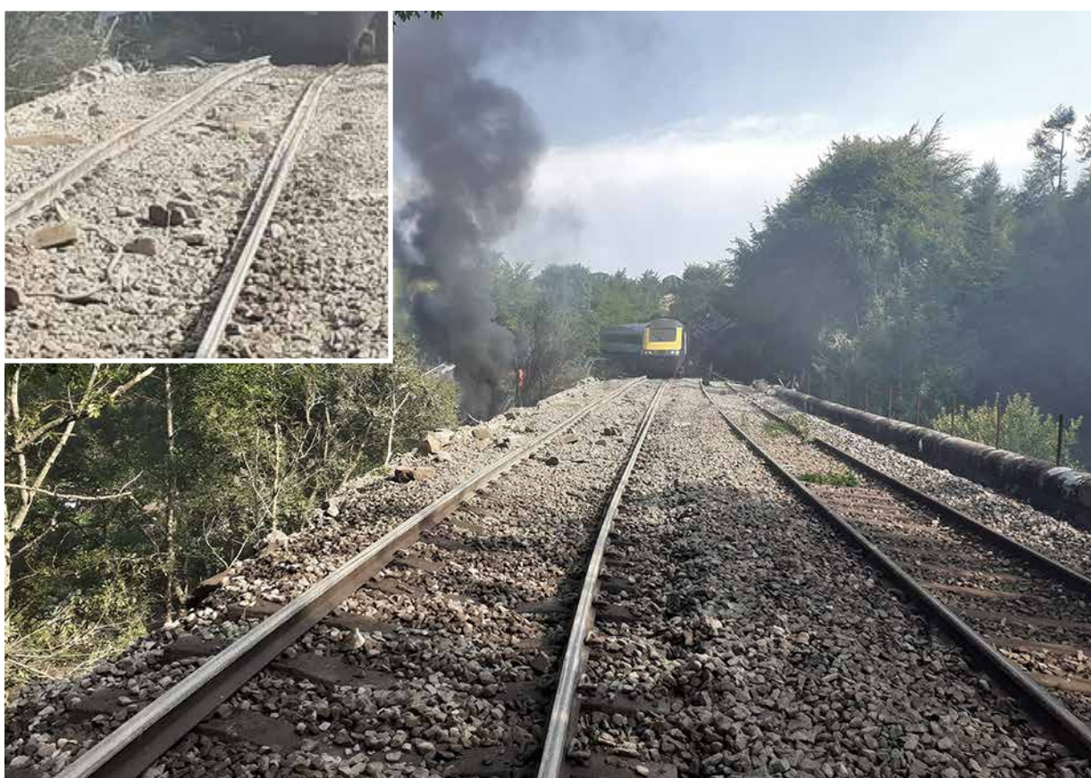
Figure F.2: Track damage across bridge 325 at 10:35 hrs on 12 August 2020 (Story Contracting)
