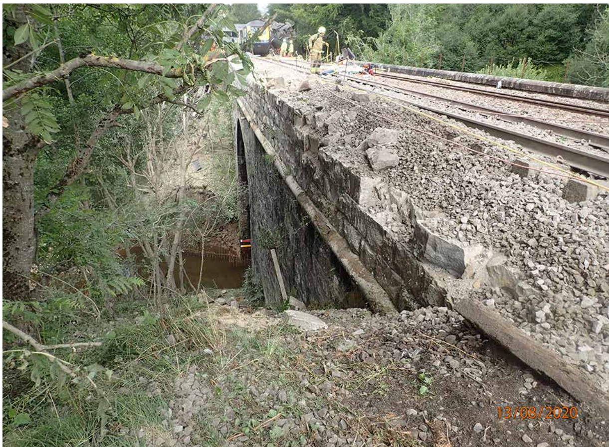
Figure F.5: Down-side parapet looking north showing damage to the parapet end
