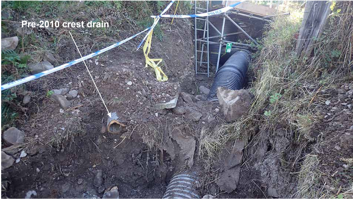
Figure G.4: Image looking upslope from near CP19 towards CP18 showing damaged end of pre-2010 crest drain close to the as-designed position of CP18. Photograph taken during post-accident investigations with scaffolding over as-built position of CP18 visible in background
