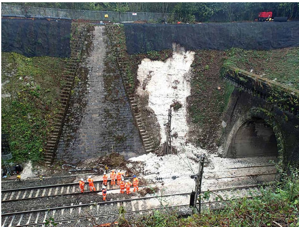
The landslip at Watford tunnel, September 2016
