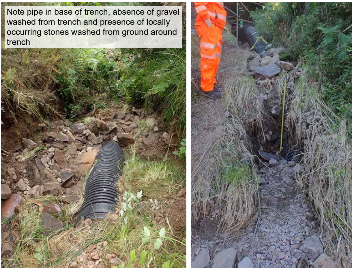
Figure 18: Washout upslope of CP18 (left image) and partial washout downslope of CP18, both images facing towards CP18
