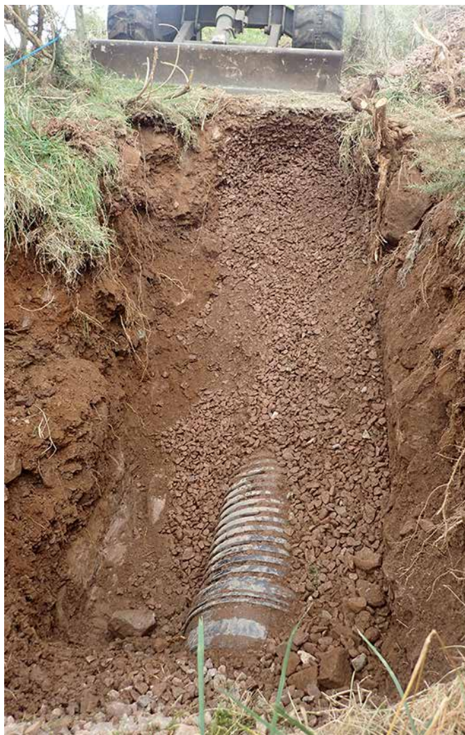
Figure 8: Gravel-filled drain close to washed out areas as exposed during post-accident excavations
