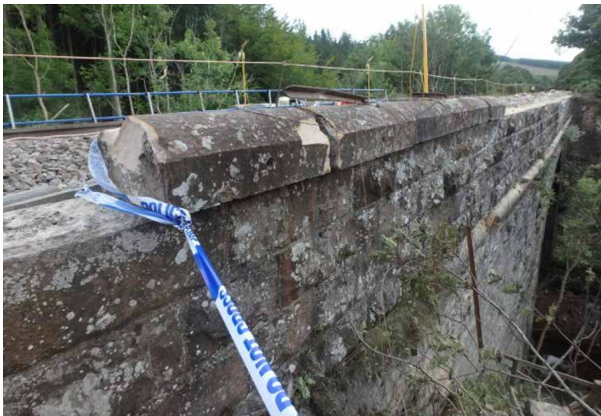
Figure F.6: Down-side parapet looking south showing remaining coping stones (Amey)
