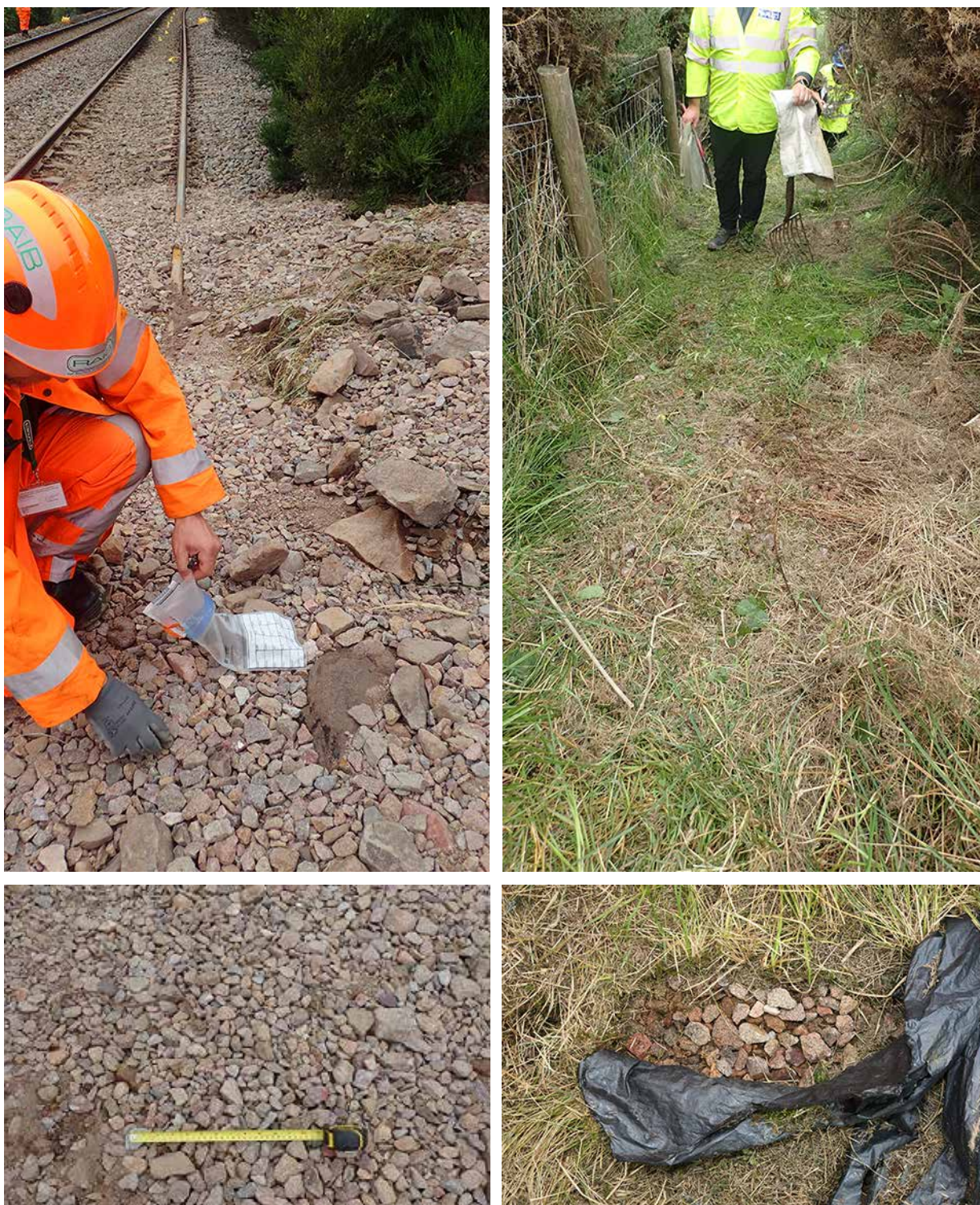
Figure 37: Landslip debris (left-hand images) and undamaged area of 2011/12 drain between washout and CP16. Surface of drain, probably protected by discarded plastic sheet since around the time it was constructed, shown in lower right image (Police Scotland)
