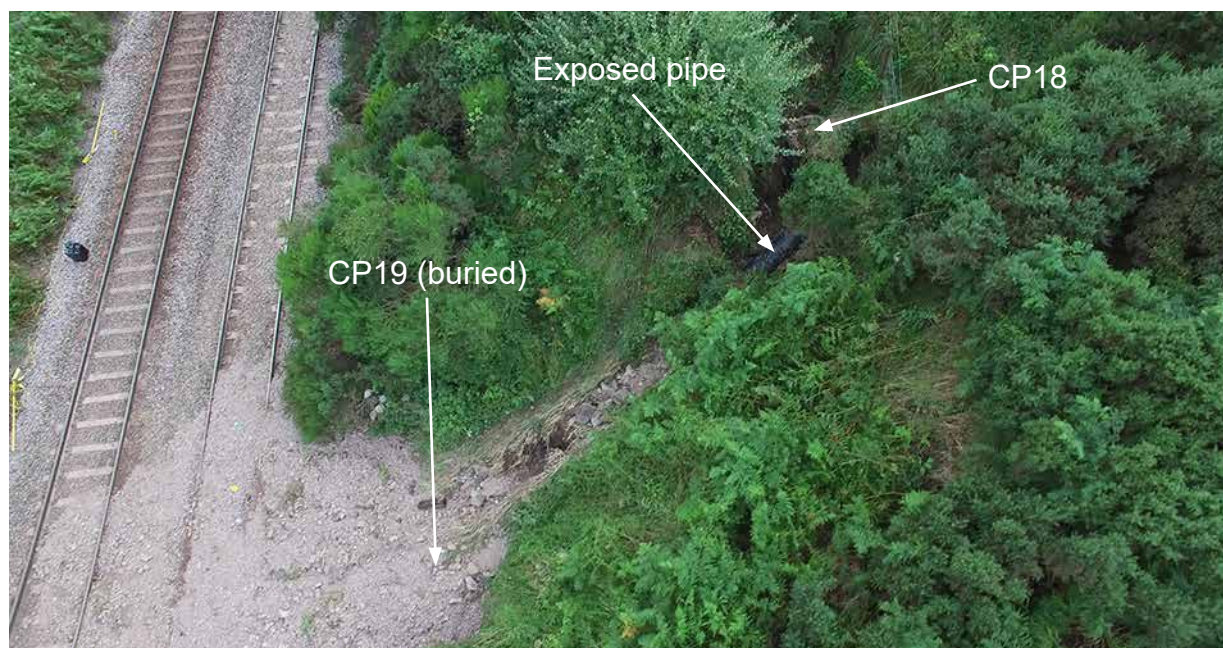
Figure 4: Washout debris on the track
