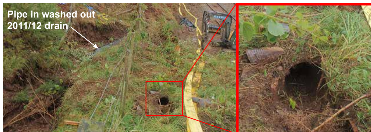
Figure G.3: Break in pre-2010 crest drain near top of washed out section of 2011/12 drain looking downslope with railway visible in top right-hand corner of image
