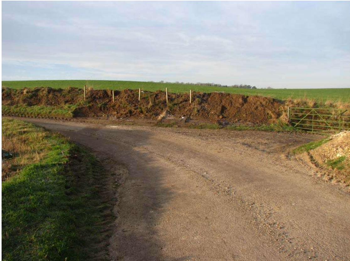
Erosion and damage caused by pipe laying in verge(Lane 9)
