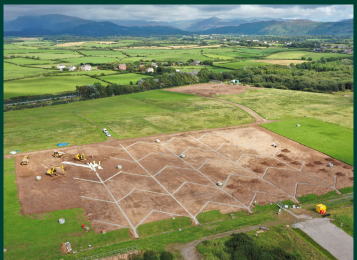
Aerial shot of the herringbone drainage installed at the Repository
