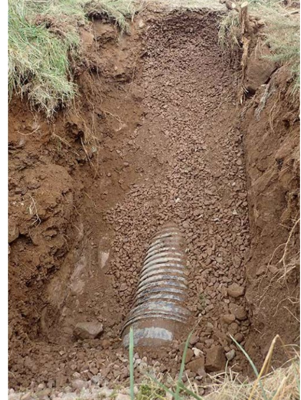
The drain's geotextile lining was omitted in the area of the washout
