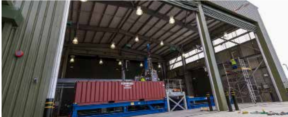
The low level waste facility in operation at Dounreay
