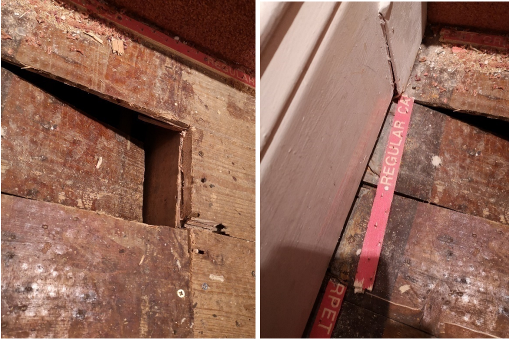
Photo 8: Floor left damaged after underfloor insulation installed. (Boiler and underfloor insulation, Owns home, AW Flexible)
