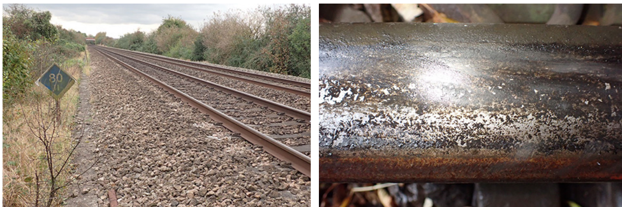
Figure 25: Location (left) and railhead condition (right) at 80 miles 40 chains.
