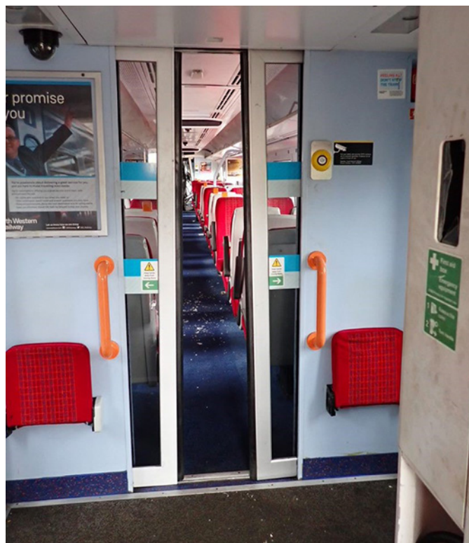
Figure 46: Image showing jammed vestibule door of the leading carriage of train 1L53.
