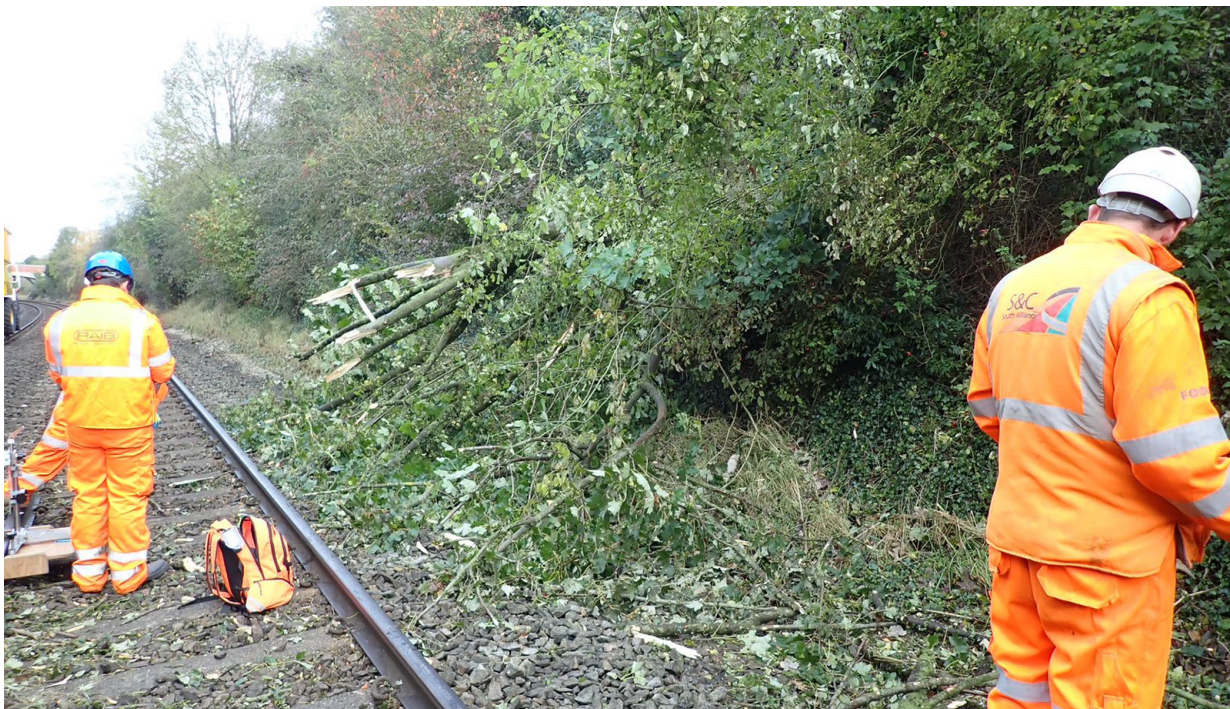
Figure 7: The tree struck by train 1L13 (post-collision) on the Down Main line looking east towards London with Broken Cross bridge in the background.
