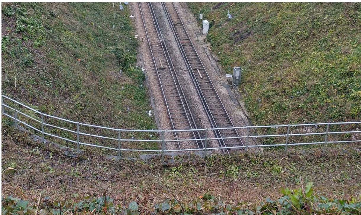
Figure 43: Image taken from a vantage point by a Network Rail MOM inspecting an HRLA site (post-vegetation clearance).
