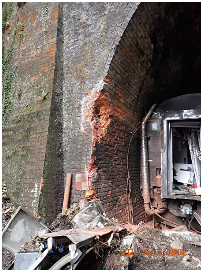
Figure 12: Impact mark from carriage A4 on facing portal wall of Fisherton Tunnel. Vestibule of A3 is visible and carriage A4 has been removed.
