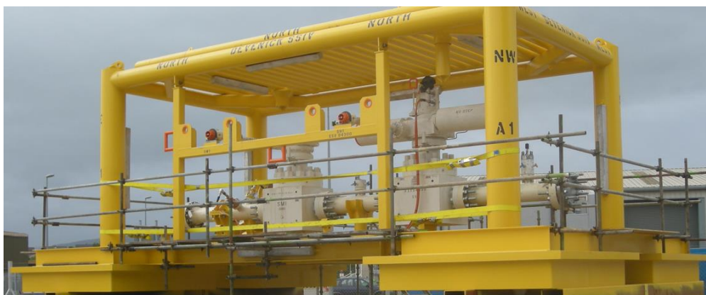
Figure 3-9 - Typical SSIV structure, analogous to that to be installed on the Teesside Pipeline
