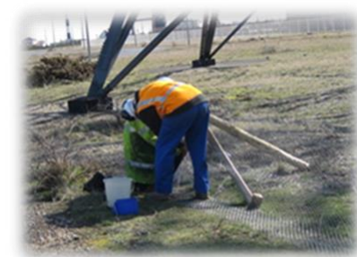
Rabbit proof fence erected on the SSSI as part of the Partnership Project
