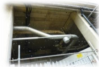
Netting to prevent bird access
