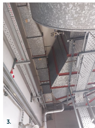
1. Typical store and associated ductwork
