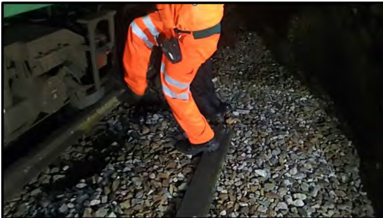
Figure 7: Still from RAIB reconstruction video showing how the detached conductor rail board can present a tripping hazard.
