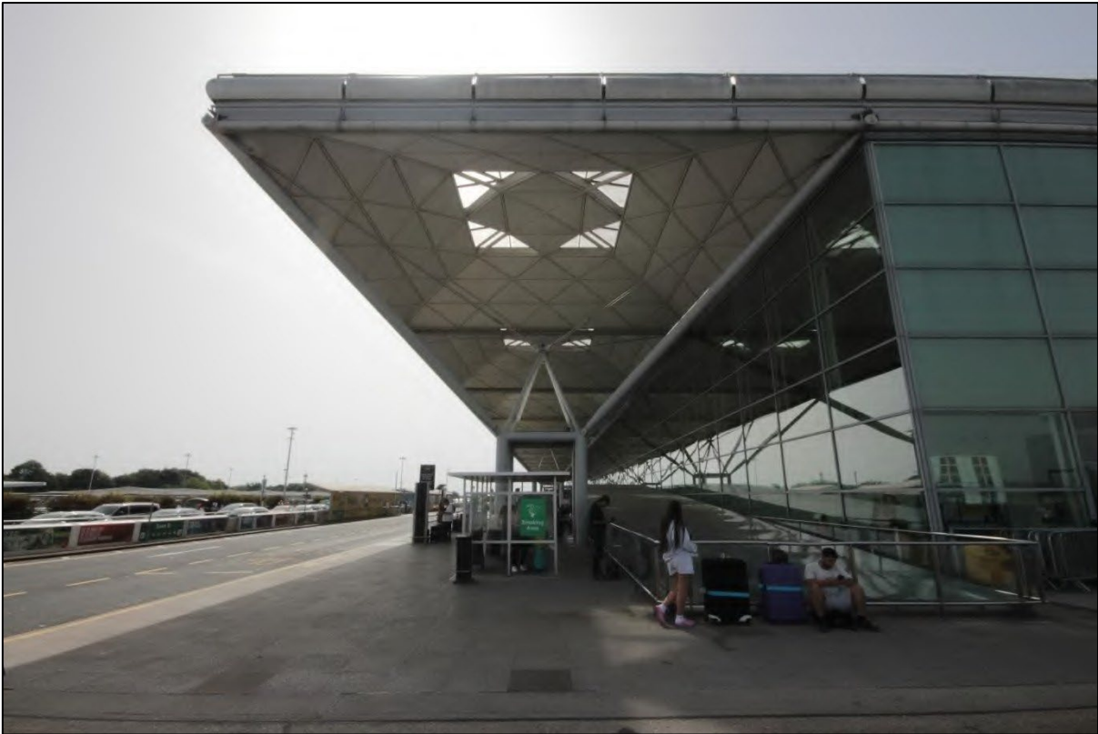
Photograph 15: View of the overhanging canopy roof on the south-eastern side of the building, taken facing south-west
