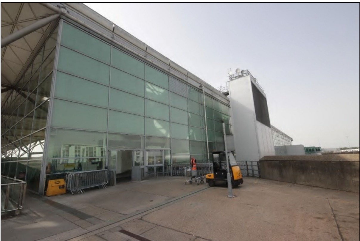
Photograph 14: View of the glazed curtain walling on the north-eastern side of the building, taken facing west
