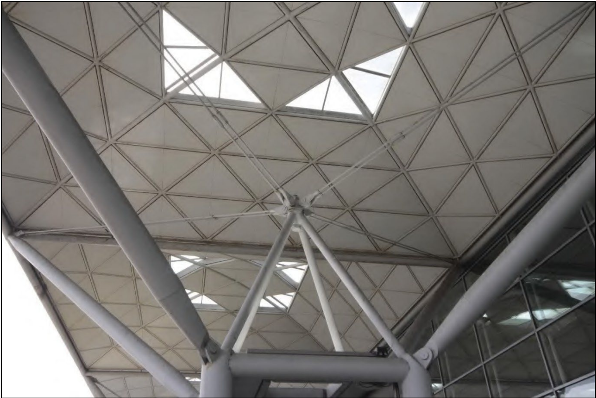
Photograph 13: View of the steel tension members and single bolt for the structural 'trees', taken facing south-west
