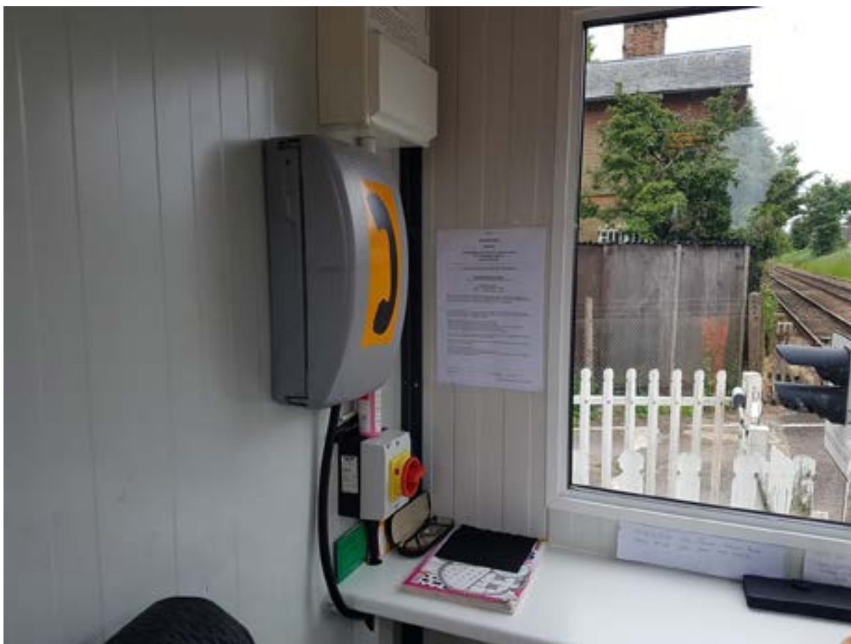
Figure 7: Crossing attendant's cabin showing gate locking switch below the telephone (installed after the incident) with view of crossing and miniature stop light equipment.
