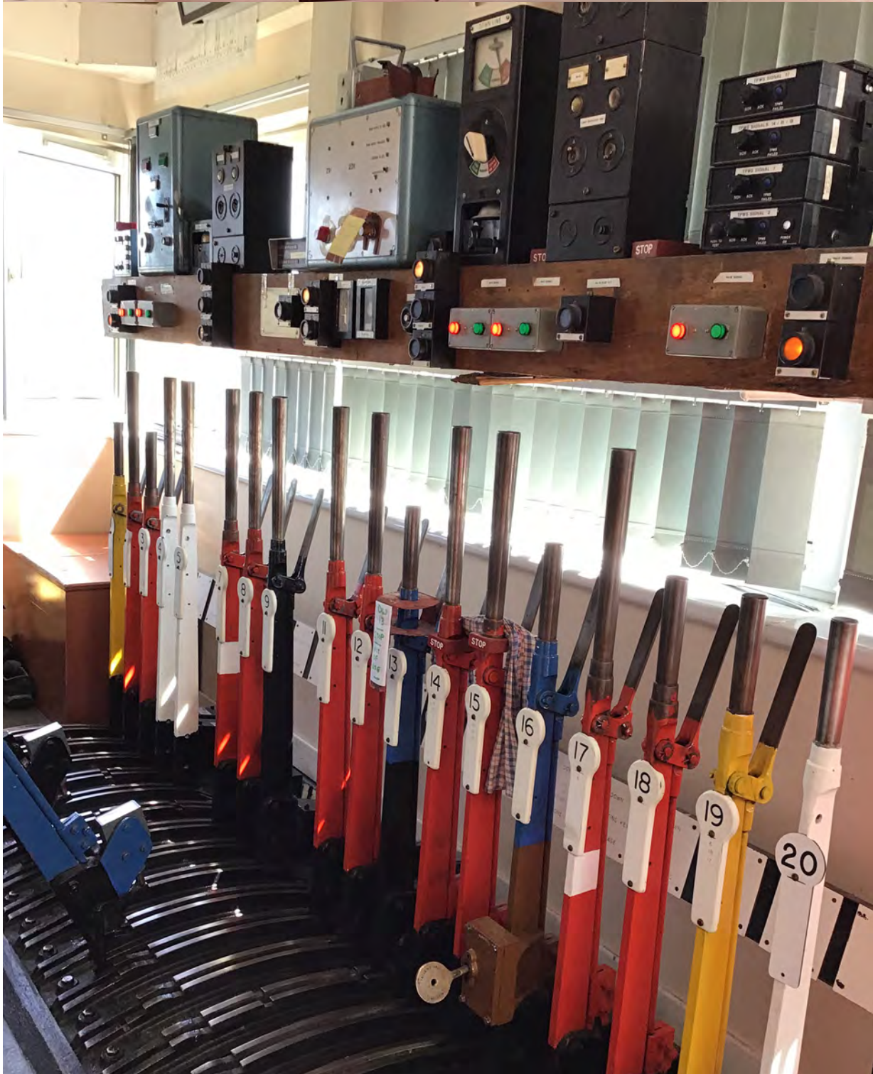
Figure 4: Signalling controls in Dalwhinnie signal box (main photograph courtesy of Network Rail)
