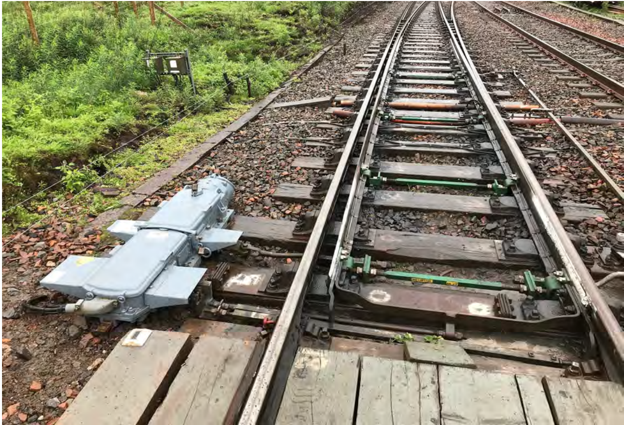
Figure 7: The newly-installed point machine at 13B point end (photograph courtesy of Network Rail)
