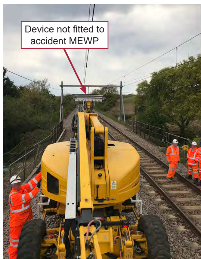
Figure 6: The view from a similar MEWP with the basket slightly raised at the accident location (in daylight)
