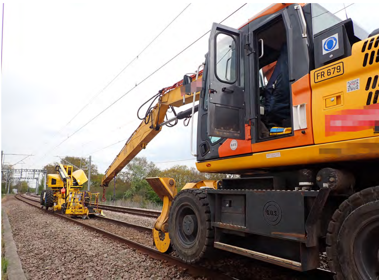
Figure 2: The rail mounted crane and elevated platform involved in the collision after being moved apart
