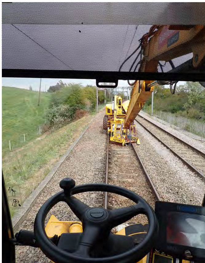
Figure 7: The view from the crane operator's seat with the sunshade drawn at the accident location (in daylight)
