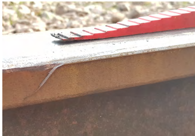
Figure 8: Wheel mark on the inside edge of the right-hand rail showing the first drop-in at the point of derailment (the red step gauge is only present to indicate the point of derailment)
