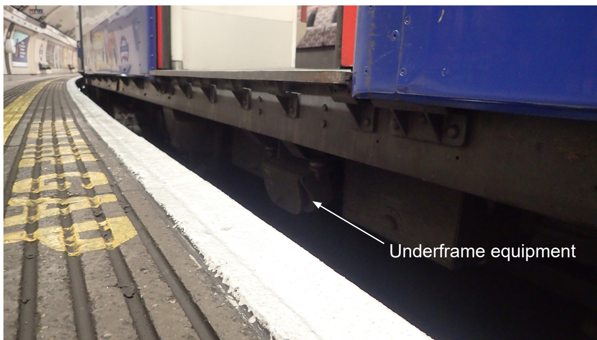
Figure 8: Proximity of under-train equipment to platform edge
