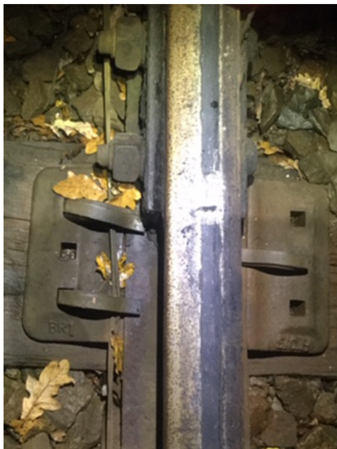
Figure 8: The railhead on approach to Norwich Road after the incident on 24 November 2019 (courtesy of Network Rail)
