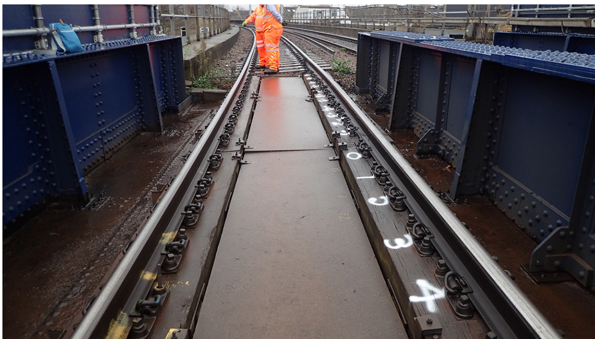
Figure 32: View of bridge 456 deck following the accident, but before the walkway was removed. With the walkway in place, the inside faces of the longitudinal timbers were not visible for inspection.
