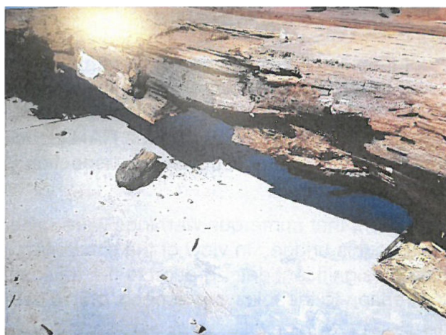
Figure 2: Condition of longitudinal timber on removal
