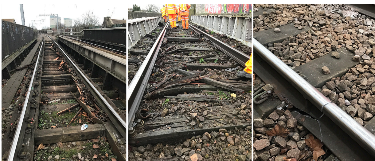
Figures 9, 10 and 11: Examples of track damage between point of derailment and location where train stopped
