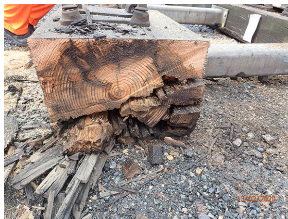
Figure 19: Section through timber 2L immediately before the point of derailment
