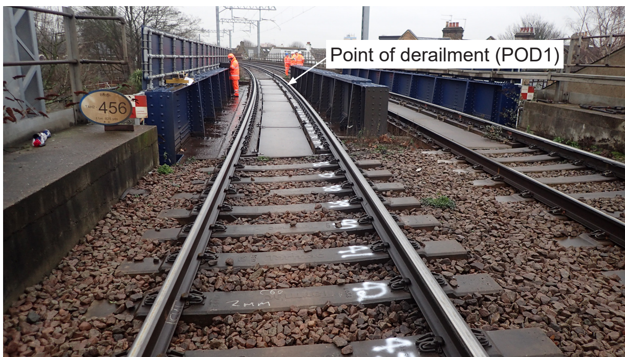
Figure 5: Bridge 456 following the accident but before removal of the deck walkway
