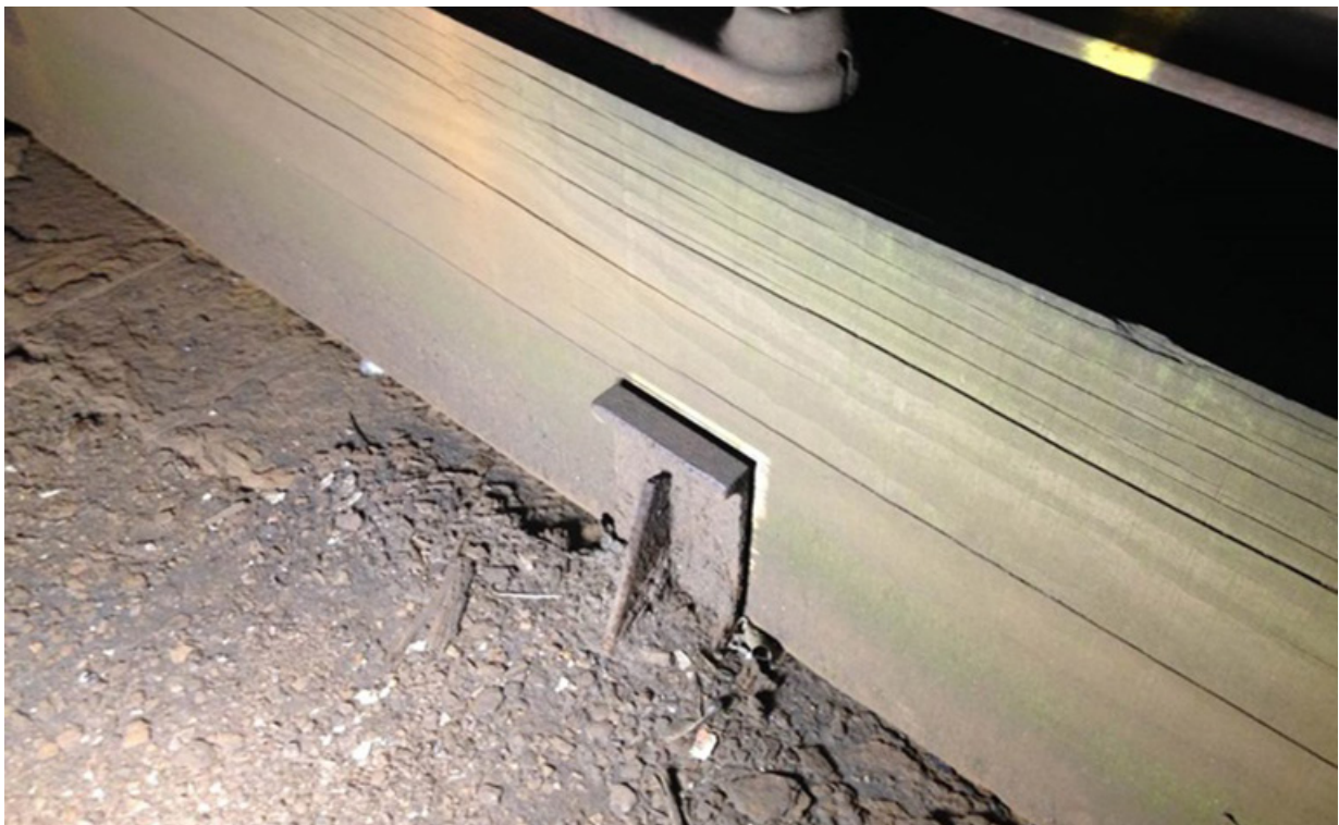
Figure 22: Photograph from detailed inspection report dated 7 June 2018 showing a restraining cleat and rust flakes on the bridge deck prior to deck refurbishment (courtesy of Network Rail)
