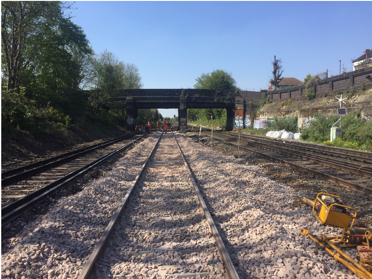
Figure 6: Train 6J91 within worksite B on the down Brighton fast line at Thornton Heath
