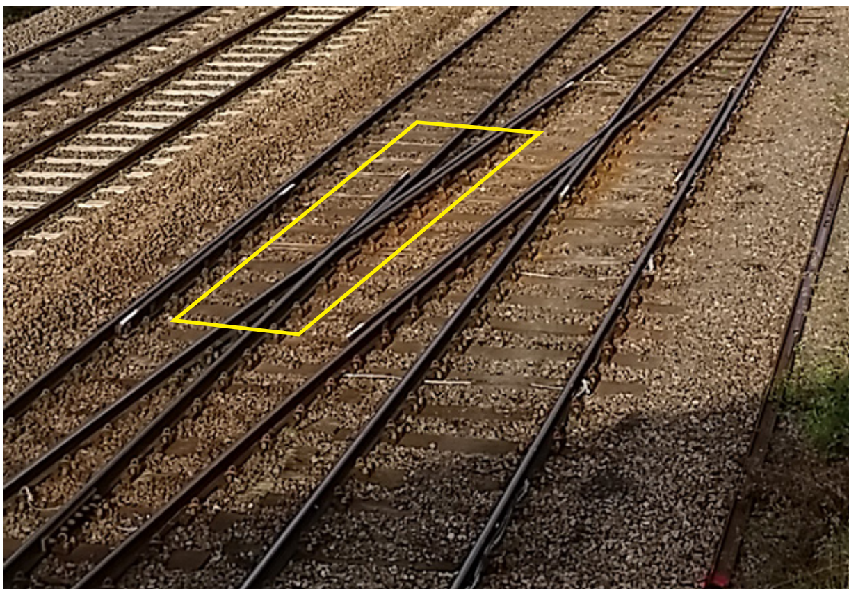
Figure 3: Photograph of a crossing within a set of points
