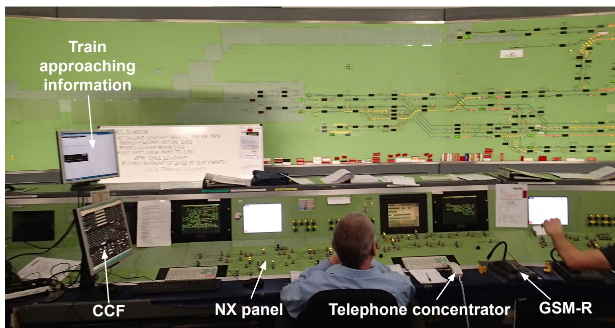
Figure 10: Panel 5 at London Bridge signal box showing the arrangement of the control, information and communication equipment
