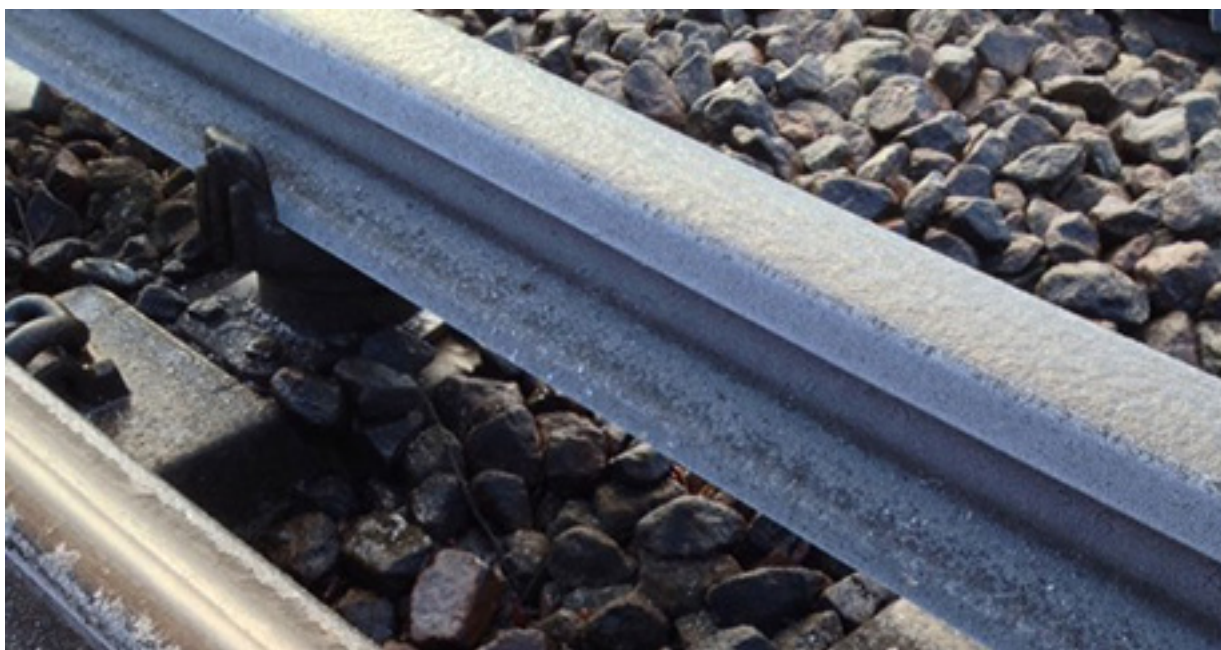
Figure 16: Typical ice and frost formation on the surface of a conductor rail (image courtesy of Network Rail)
