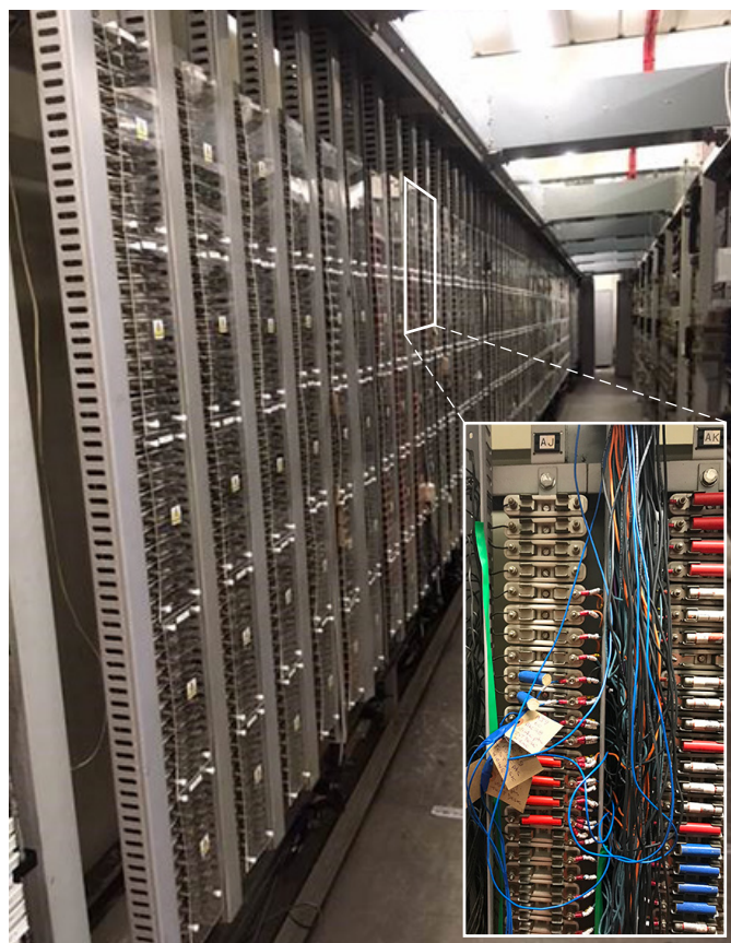
Figure 10: Waterloo relay room with inset including connections from 1524 points and associated fuse holders as detailed in figure 19
