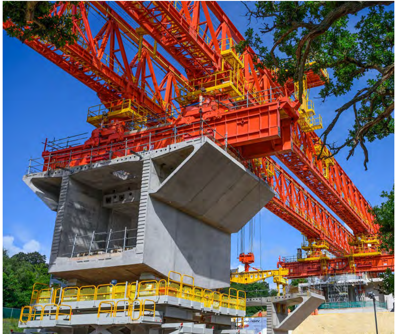
Dominique, HS2’s launching girder, placing pre-cast concrete sections into position for the Colne Valley viaduct.
