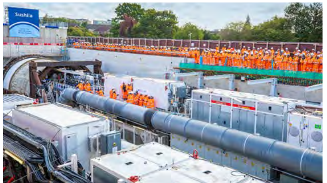
The work to build 13 miles of tunnels under London begins as the first tunnelling machine sets off from West Ruislip.
