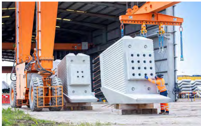
The first pre-cast segments for the Thame Valley viaduct at a factory in Kent.
