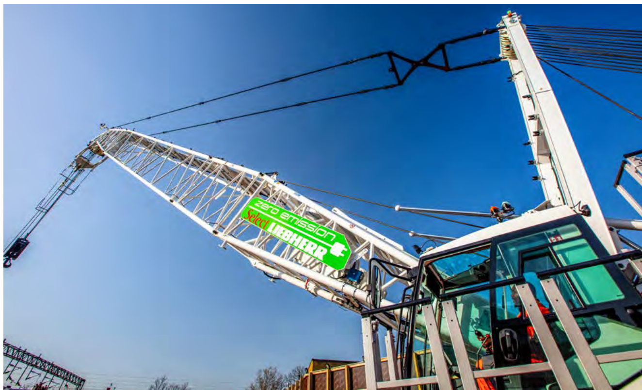
An electric crawler crane at Old Oak Common station, south Kilburn, London.
