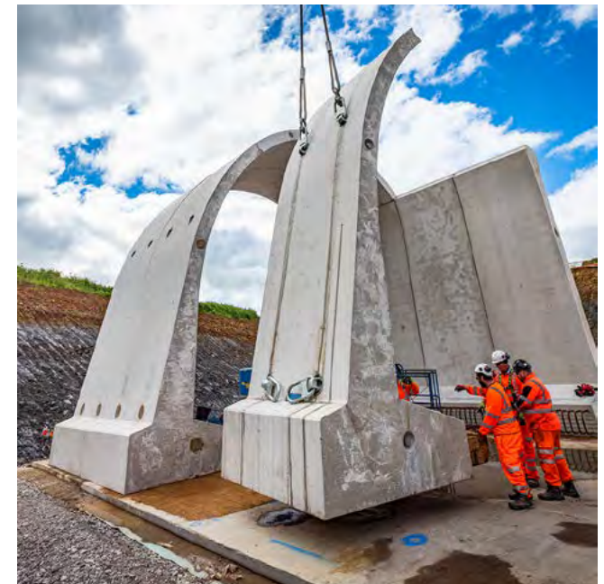
Pre-cast concrete segments being craned into place for the green tunnel at Chipping Warden.
