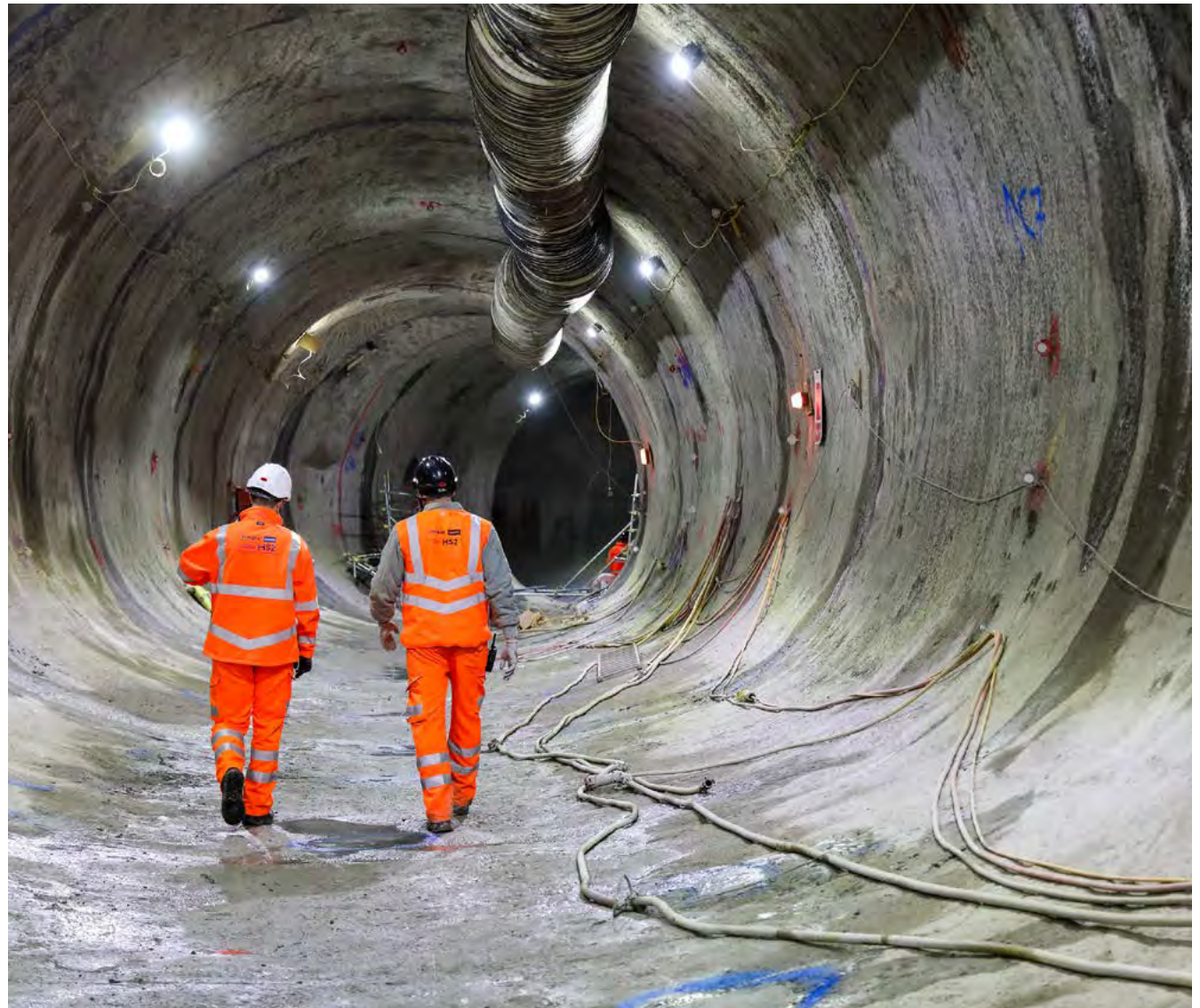
The traction substation tunnel at Euston.
