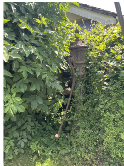
Figure 23B Close up image of Pump at Pippins (source: Google Maps)
