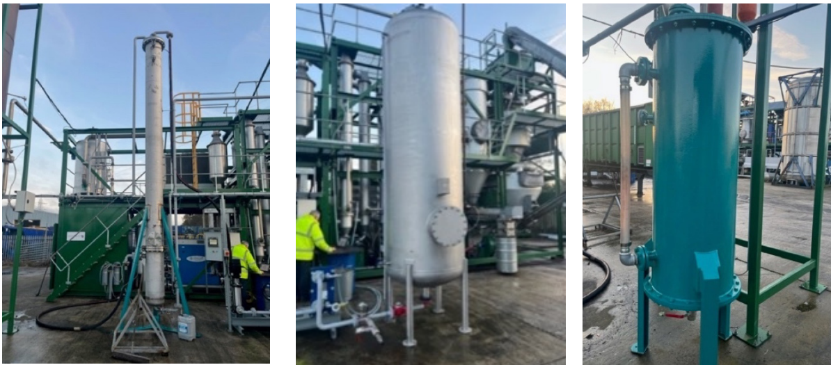
Figure 2 The \text{CO}_2 scrubbing column (left), water regeneration vessel (middle) and flare pot (right) fabricated and mounted in position.
