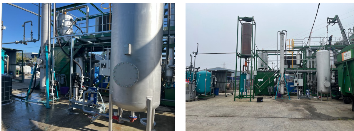
Figure 3 Arrangement of the final CSS Gasifier-500 and carbon capture pilot plant.
