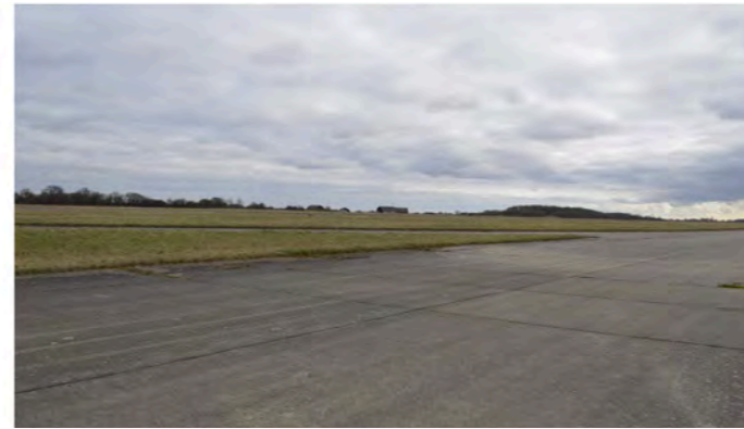
2. View to the north east across the runway looking towards the Dutch Barns and Park Wood.
