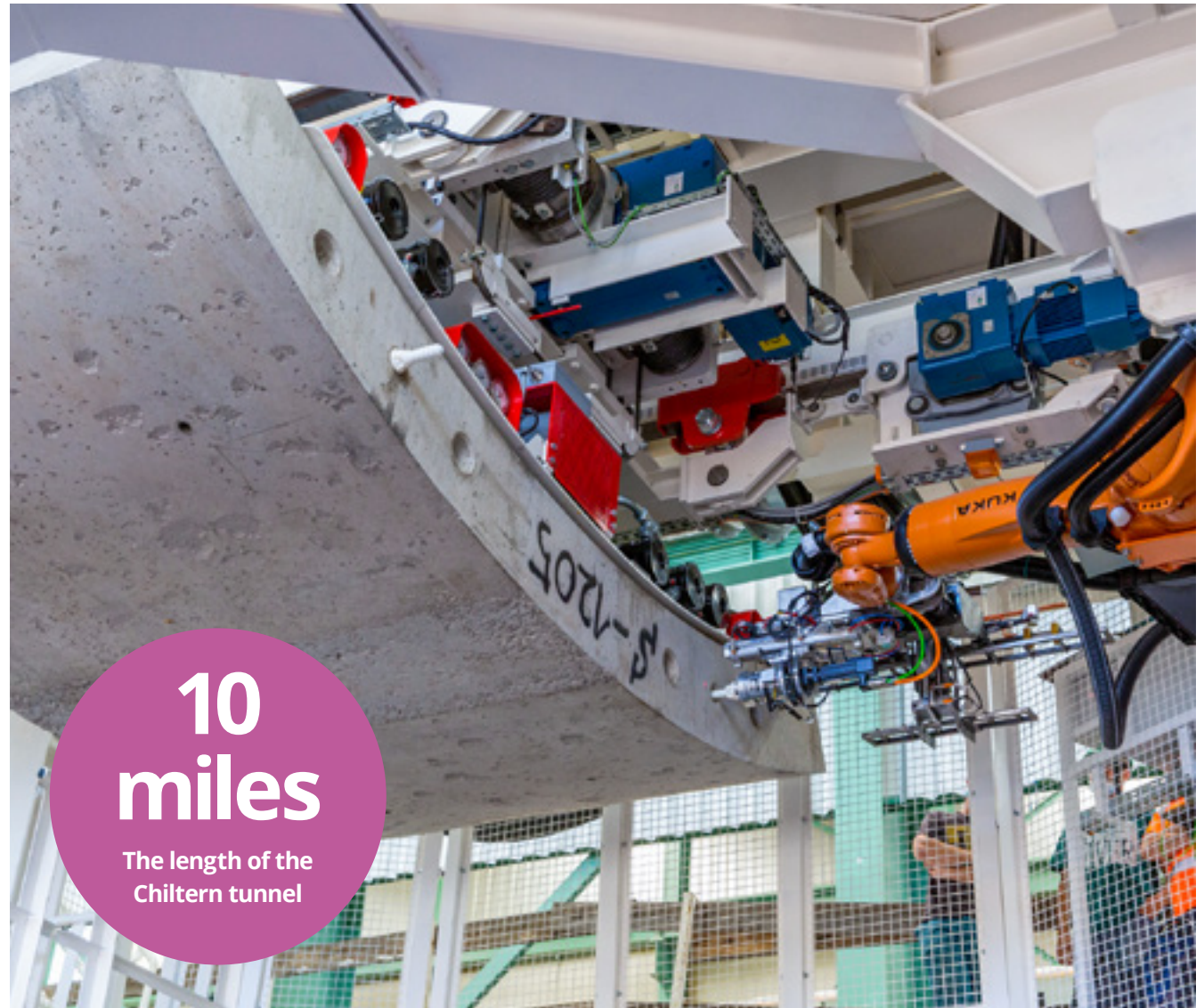
Part of the concrete sleeve being placed in position by a tunnel boring machine.
