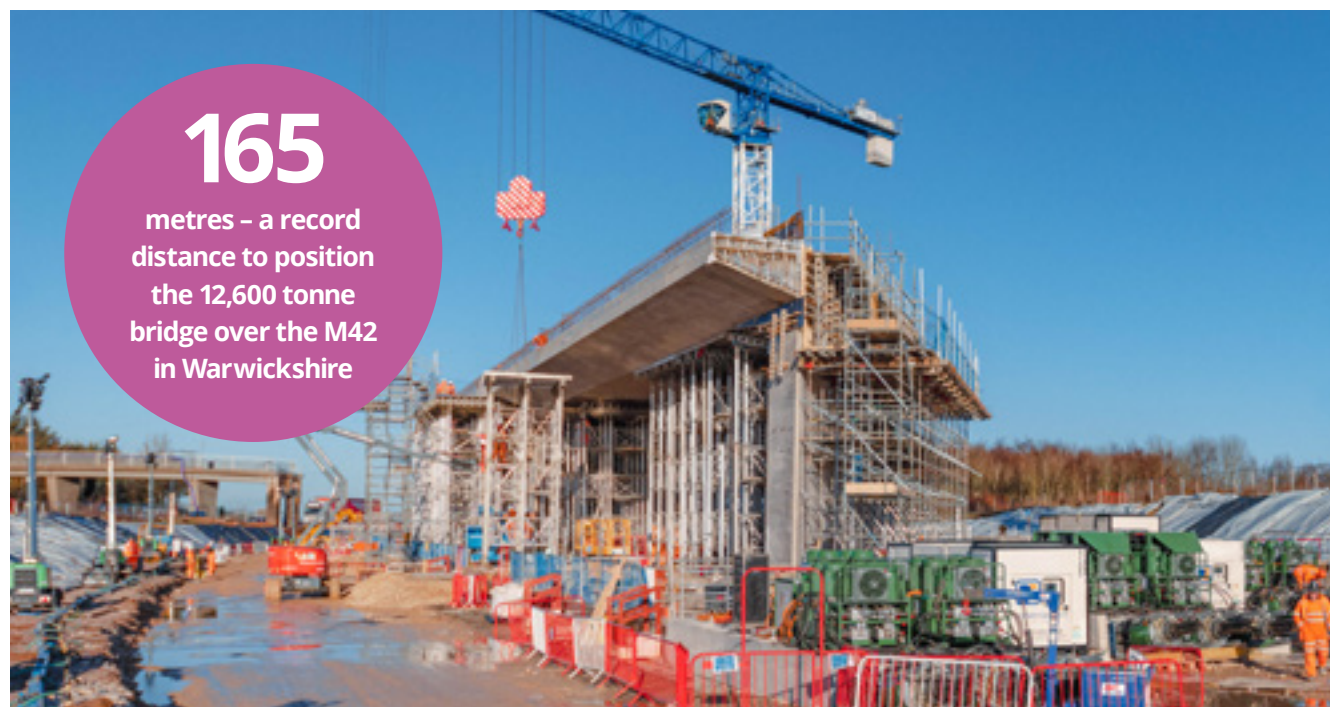
The Marston Box bridge structure was fully assembled on land next to the M42 motorway, prior to being installed.
