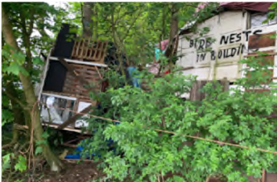
Photograph of NE structure on 10.05.2022, showing collapsed "east wing":
