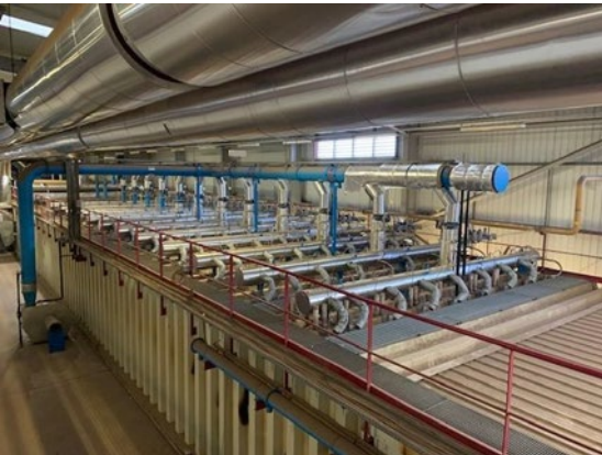
New Insulation being installed on the top combustion air system to reduce heat loss and prevent contact with hot surfaces
