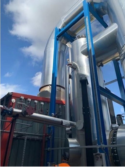
New external heat exchanger connected and in operation
