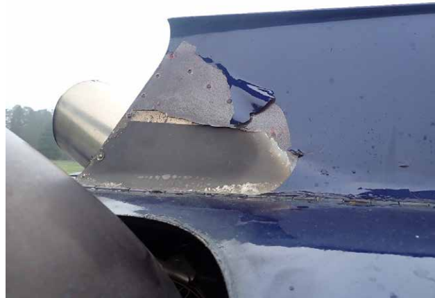
Paint blistering on engine cowling adjacent to right engine inboard exhaust tube
