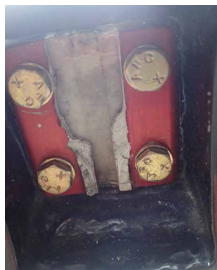
Parts of the failed centre hinge attachment for the right aileron before removal from wing
