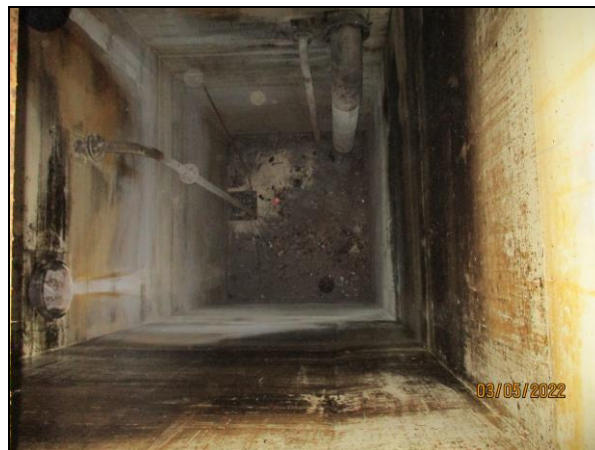
Photograph 6: Wet sump before decontamination
