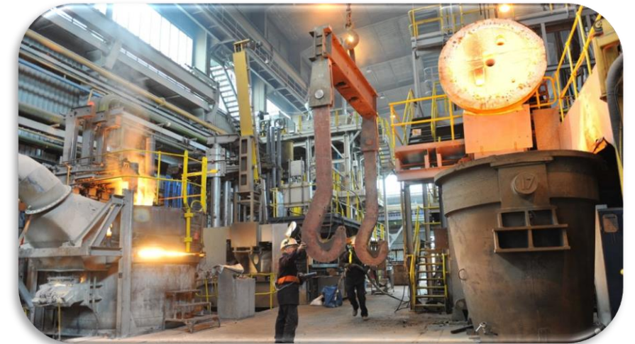
The pre-heat ladle at the MPI's Normanton Plant - MPI [Primary end-user stream 2B]
