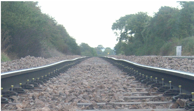
An example of poor track geometry which resulted in derailment of a freight train.
