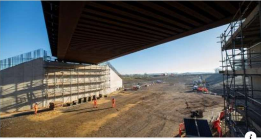
NEWCIVILENGINEER.COM HS2 contractors build key East West Rail bridge in Buckinghamshire The bridge will carry direct EWR services between Oxford and Cambridge. Engineers working f...
