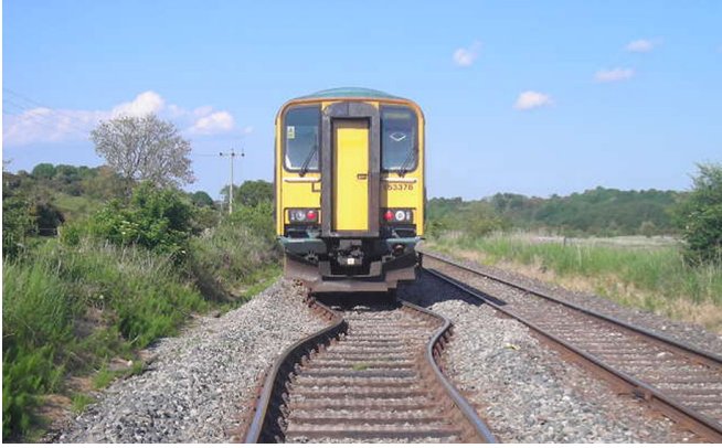
Severe track buckle at Cummersdale.
