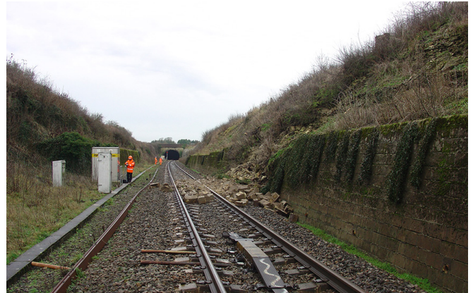
Collapsed wall following landslip at Kemble.
