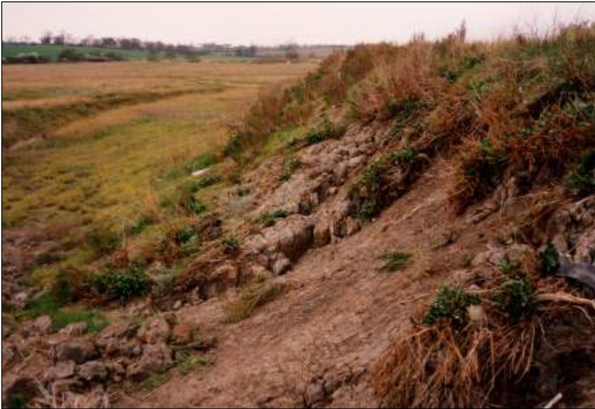
Figure 26 - Photo showing grass erosion due to overtopping Photos source: Environment Agency (2007).
