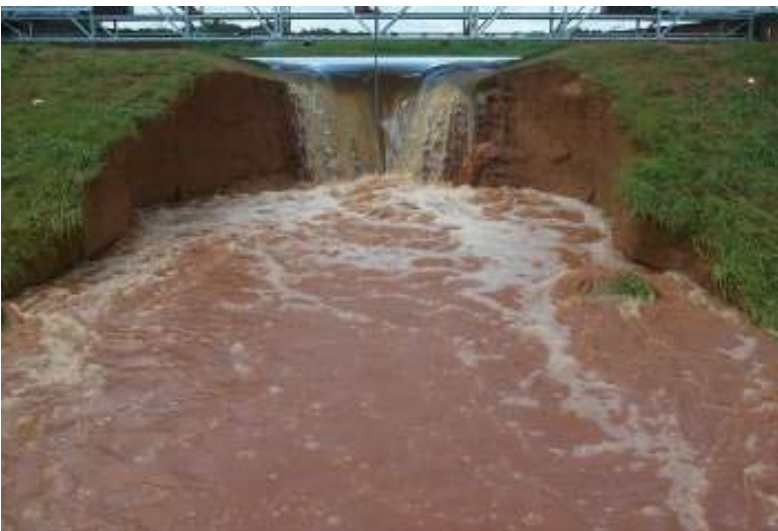
Figure 8 - Image of breach formation as headcut enters the reservoir
