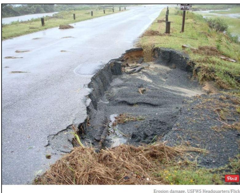
Figure 29 - Photo showing road cover affecting embankment erosion process
