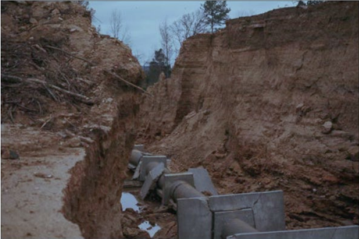
Figure 24 - Photo of transitions as a focus for erosion (Photo D Bowles/USBR/USACE)
