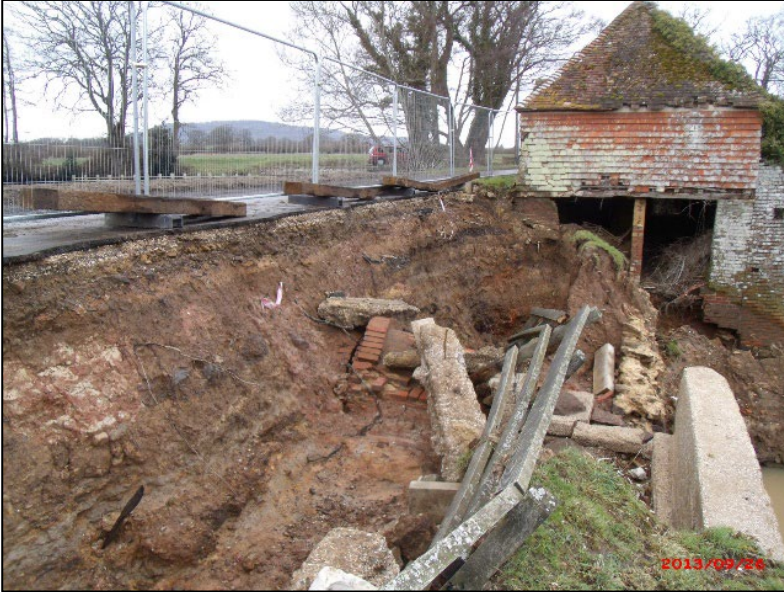
Figure 30 - Photo showing overflow erosion at a small dam in Surrey in the December 2013 floods (Incident 388 in the EA database)
