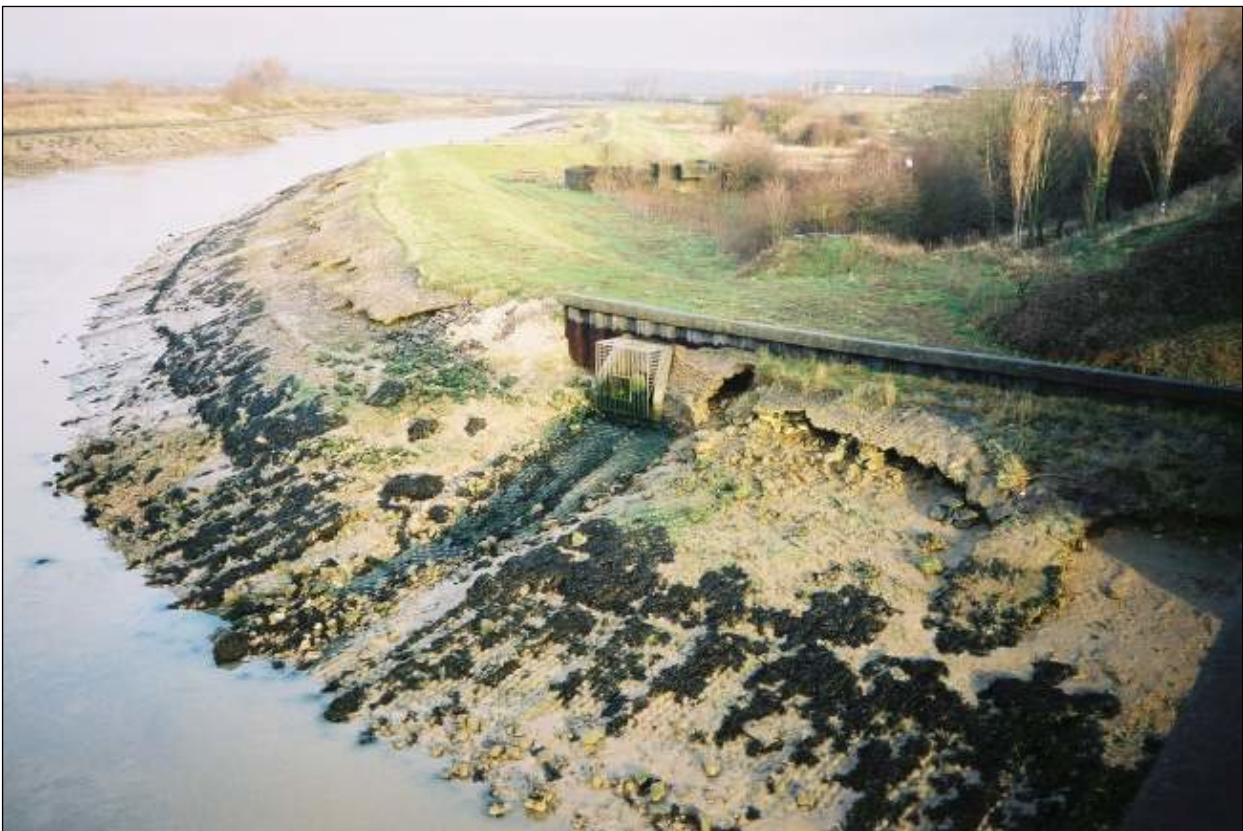
Figure 23 - Photo of erosion as a result of a transition (Photo – MW Morris)
