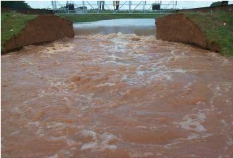
Figure 9 - Image of breach expansion during reservoir drawdown
