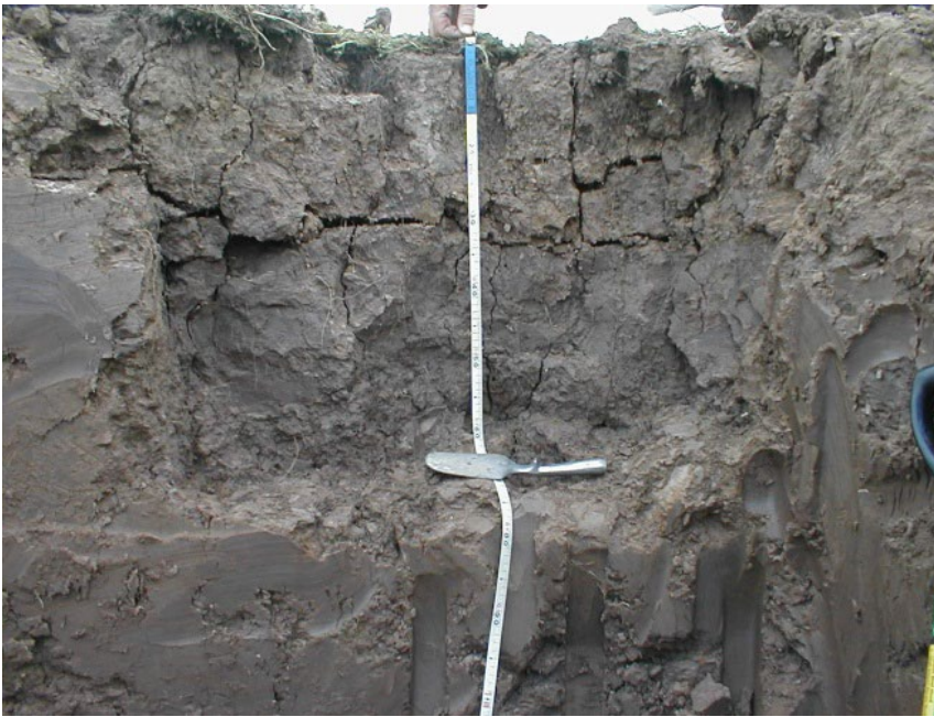
Figure 28 - Photo showing embankment fissuring: depth of cracking in original embankment at Thorngumbald Photos source: Dyer and others (2007).
