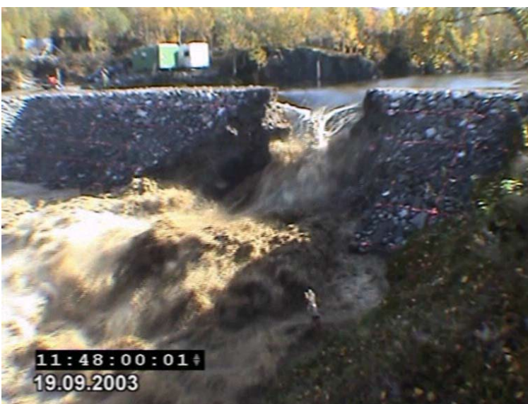
Figure 13 - Image of continued surface erosion, including crest erosion and some breach widening
