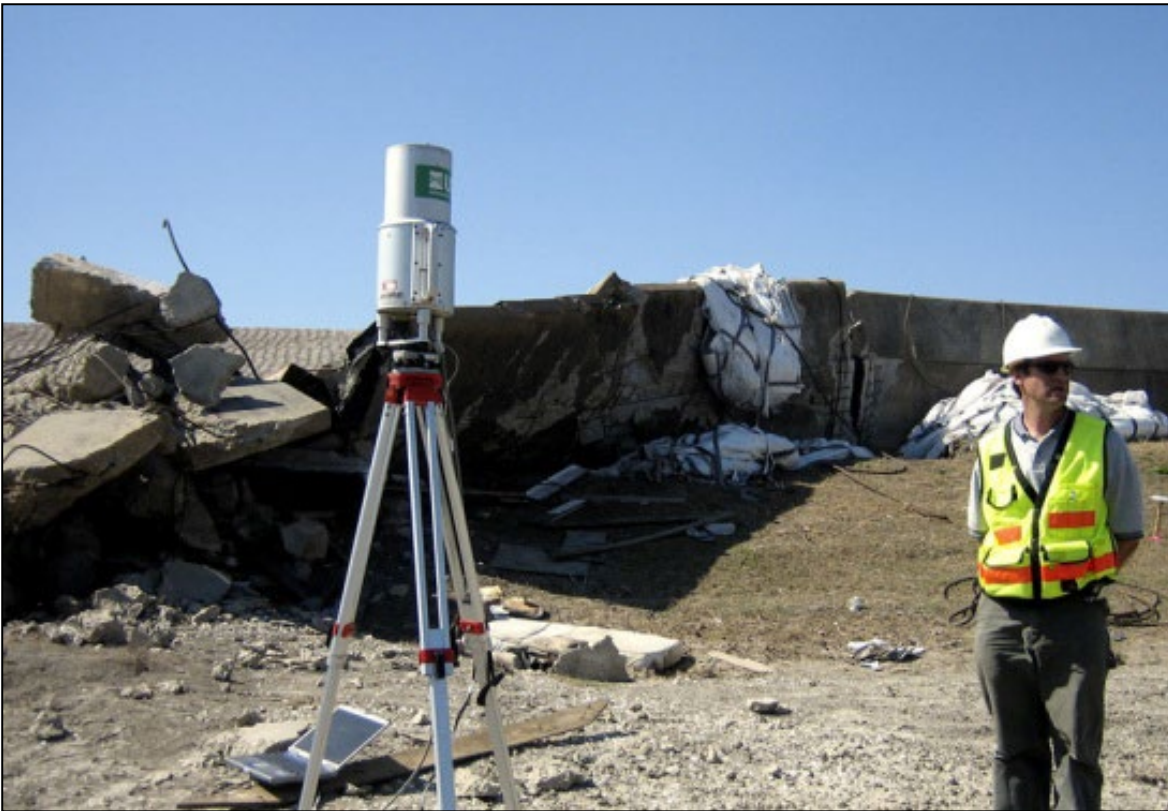
Figure 32 - Photo showing overflow damage to concrete flood walls during Hurricane Katrina
