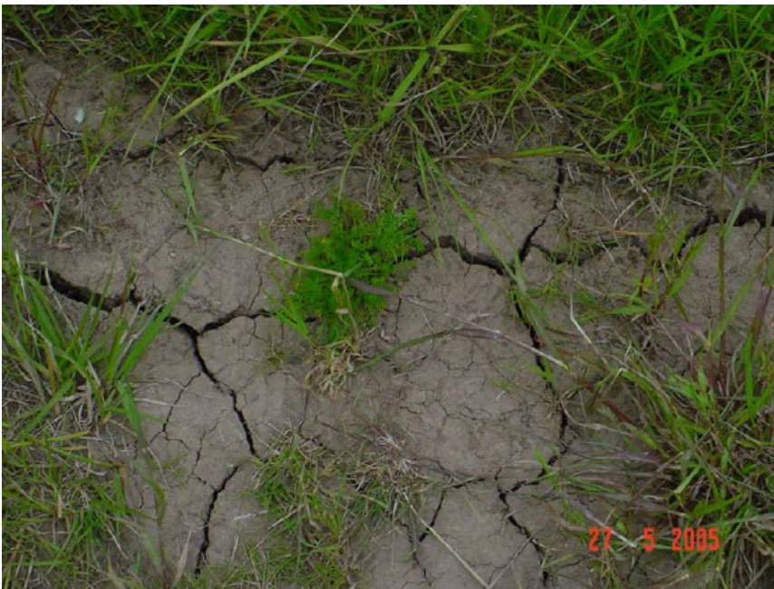
Figure 27 - Photo showing embankment fissuring: Surface cracking in new embankment at Thorngumbald Photos source: Dyer and others (2007).
