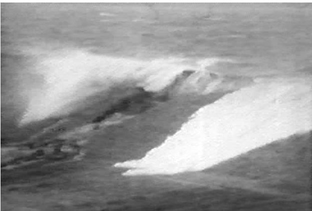
Figure 37 - Photo of erosion of landward face of a coastal levee
