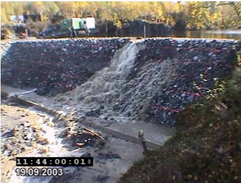
Figure 10 - Image of initial overflow and surface erosion
