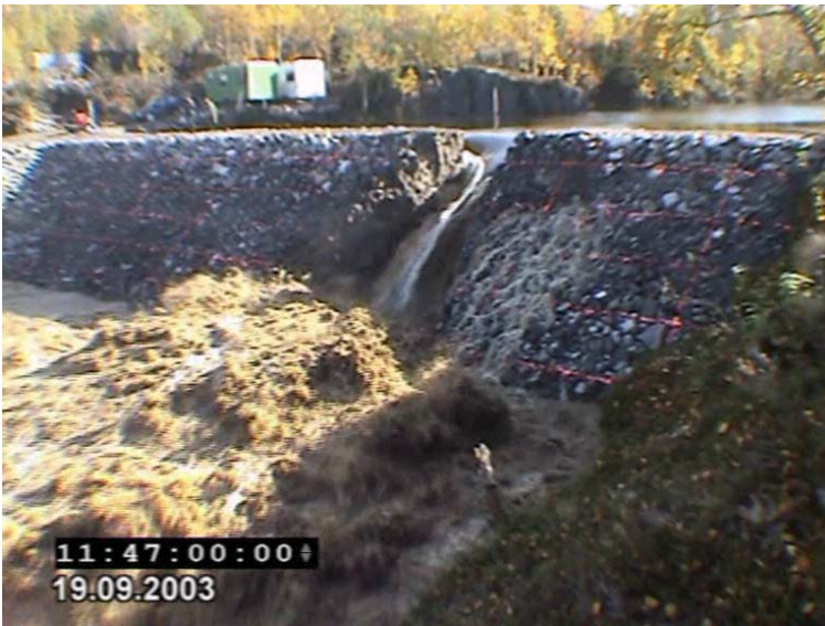
Figure 12 - Image of continued surface erosion, including crest erosion
