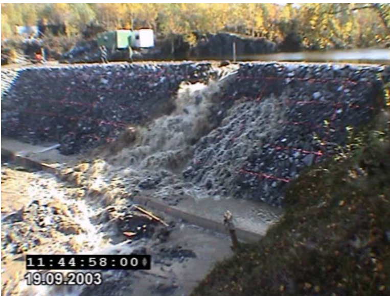
Figure 11 - Image of continued surface erosion, including crest erosion
