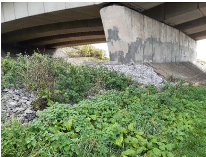
Figure 1.3 Third party Type 4 (revetment) transition not identified by interrogation of the Environment Agency AIMS database
