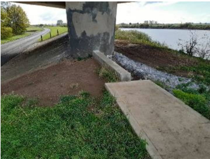
Figure 6.29: Example of poor grass caused by shading and possibly impeded root formation, M180 crossing along Tidal River Trent, 2020
