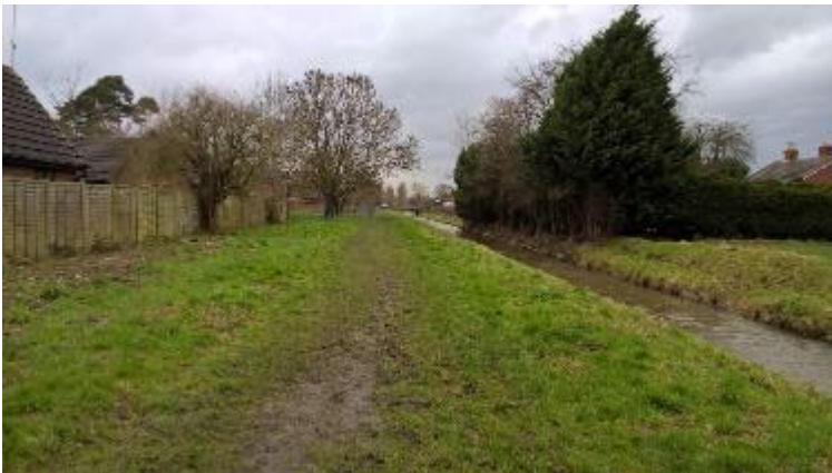
Figure 6.39: Rutting and furrowing on embankment crest, Leominster (River Lugg), 2017
