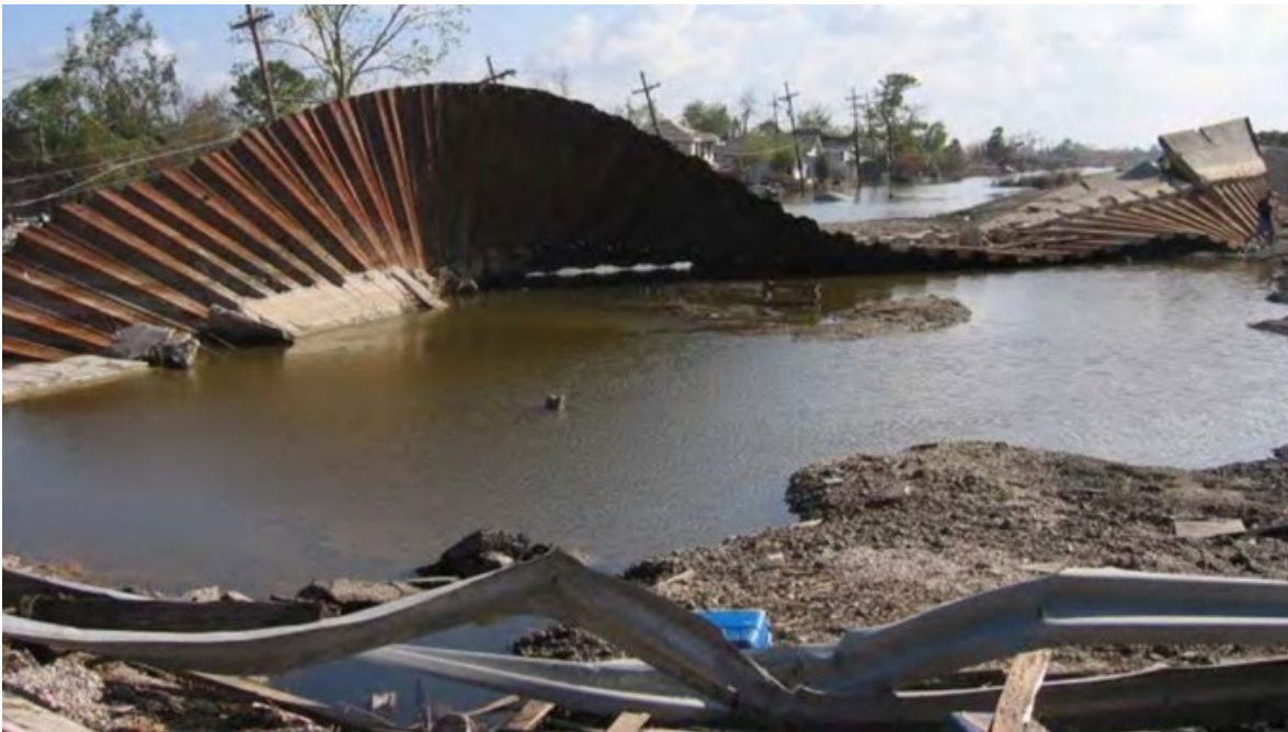
Figure 6.24: I-walls failed during Hurricane Katrina due to stiffness incompatibility
