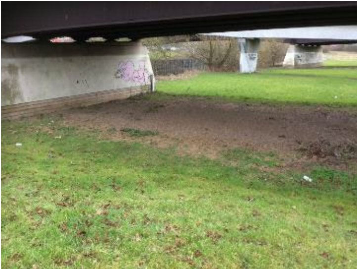
Figure 6.28: Example of poor grass caused by shading, Alney, 2018
