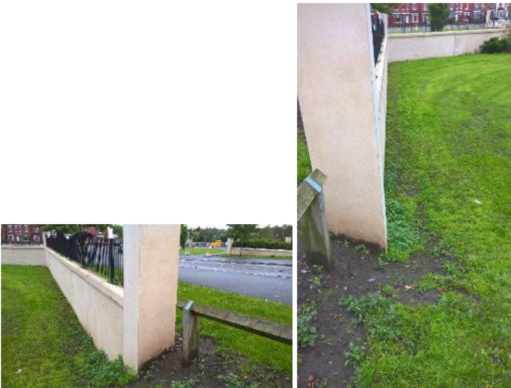
Figure 6.36: Example of impeded maintenance causing vulnerability to surface erosion, Victoria Park Warrington, 2019
