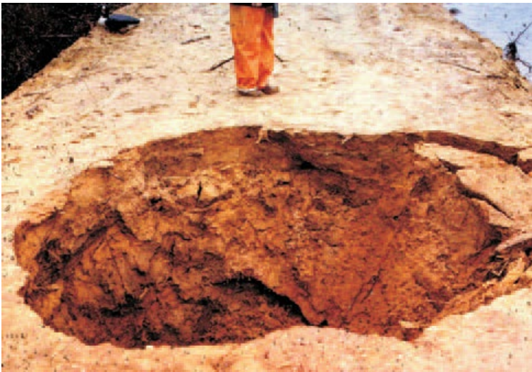
Figure 6.32: Embankment collapse (possibly poor compaction coupled with seepage – FEMA
