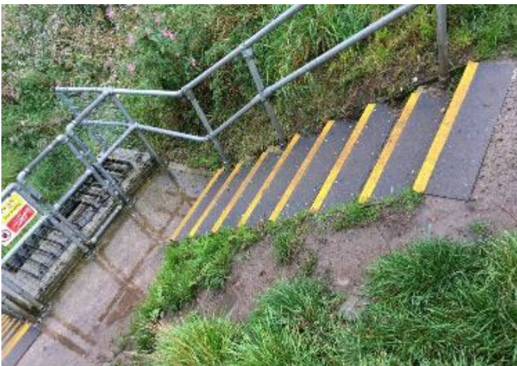
Figure 6.40: Handrail and restricted access on to the structure has promoted preferential path alongside the steps (likely due to downhill cycling), Fletcher Moss Park (River Mersey), 2019
