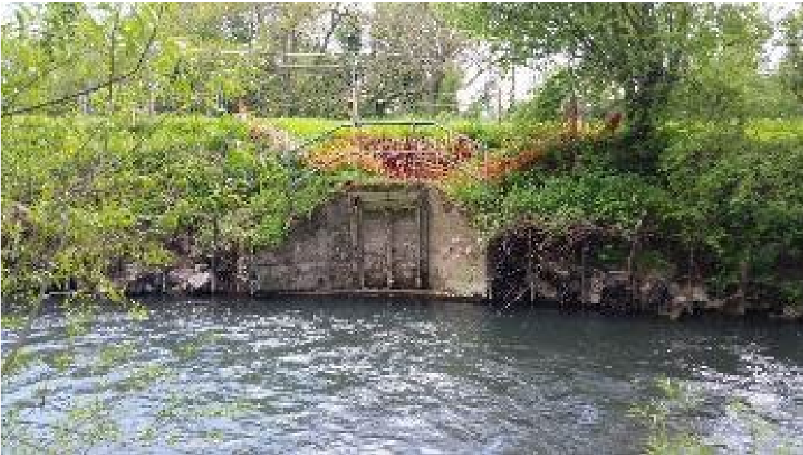
Figure 6.14: Gabion baskets applied as toe protection washed away as located at vulnerable point creating irregularities, Butt's Bridge, Leominster 2018
