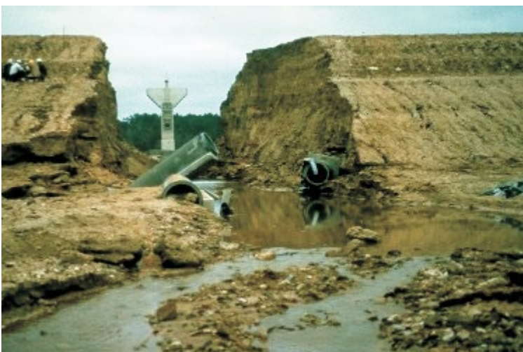
Figure 6.33: Failure due to transition, possibly caused by poor compaction FEMA 484
