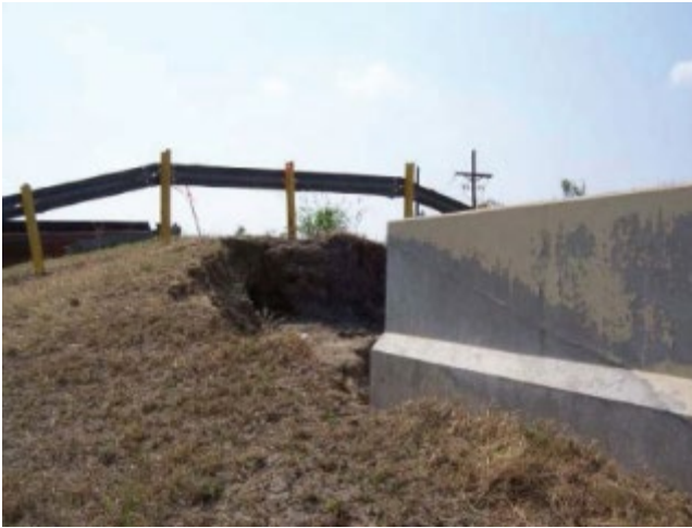
Figure 6.11: ILH Figure 9.65 New Orleans levee scour at transition with a flood wall (courtesy USACE)
