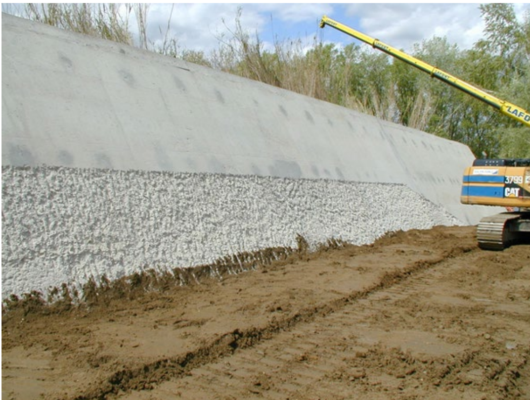
Figure 6.4: Preparation of the flood wall transition at Comps by roughening up the surface (courtesy of Thibaut Mallet; see ILH Figure 9.66)
