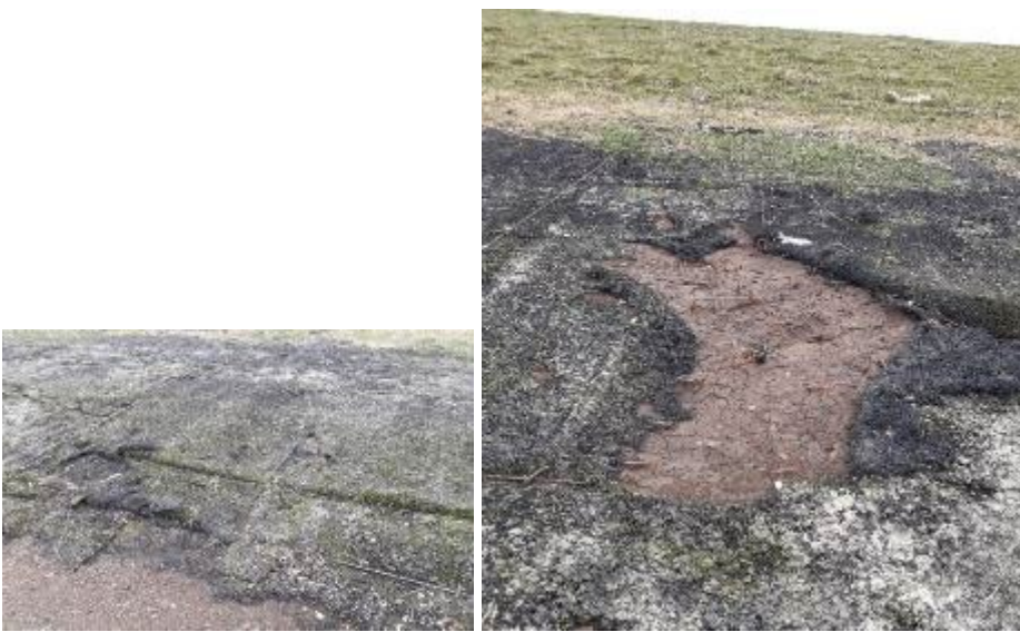
Figure 6.21: Insufficient overlap between the geotextiles on toe erosion protection, along north Kent coast, 2020
