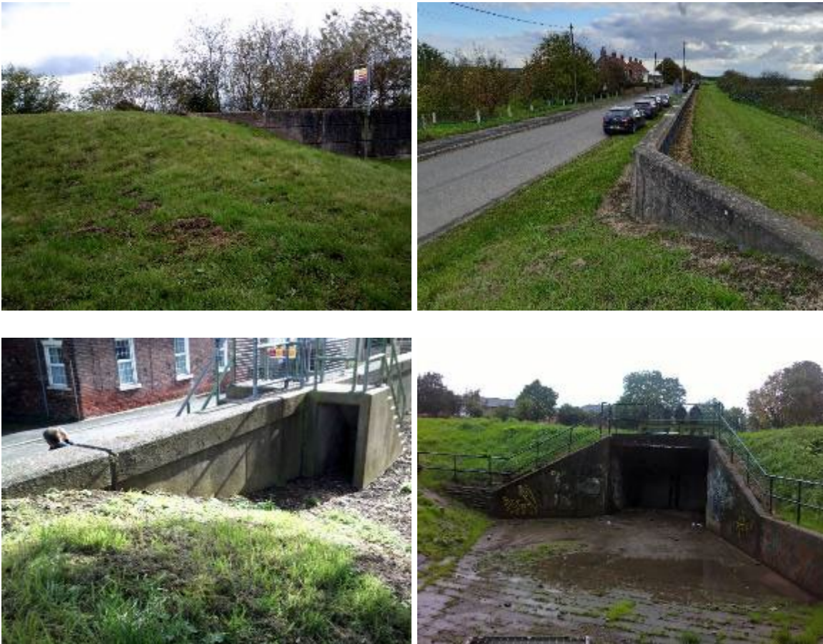
Figure 3.2: Type 1 transition examples: 3 embankment-wall transitions near East Ferry (Tidal River Trent). The bottom right picture shows a transition between an embankment and a concrete outfall structure (flood storage reservoir at Northenden Riverside Park, River Mersey)
