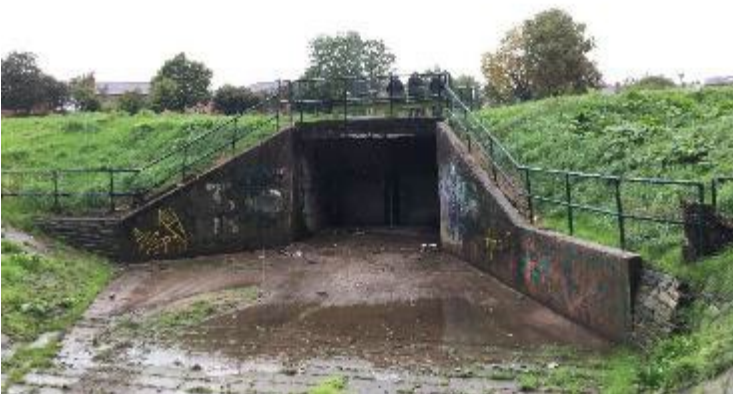
Figure 6.12: Crest level difference that could concentrate overtopping flow onto poor grass near transition, flood storage reservoir at Northenden Riverside Park (River Mersey), 2019
