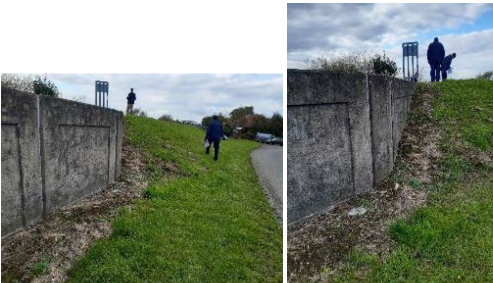
Figure 6.37: Example of impeded maintenance causing vulnerability to surface erosion, south of East Ferry (Tidal River Trent), 2020
