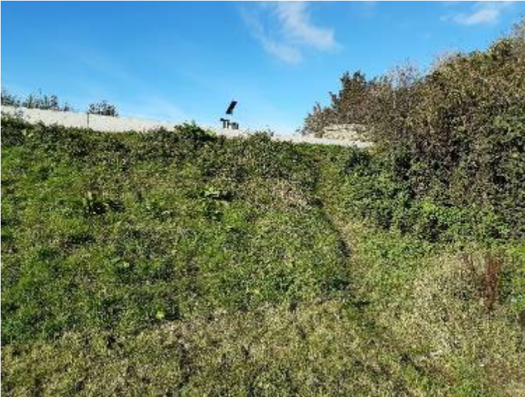
Figure 6.41: Preferential path alongside landward slope at overgrown transition near Scunthorpe (Tidal River Trent), 2020
