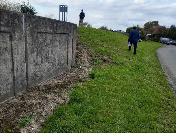
Figure 4-2: Poor maintenance regime causing vulnerability to surface erosion
