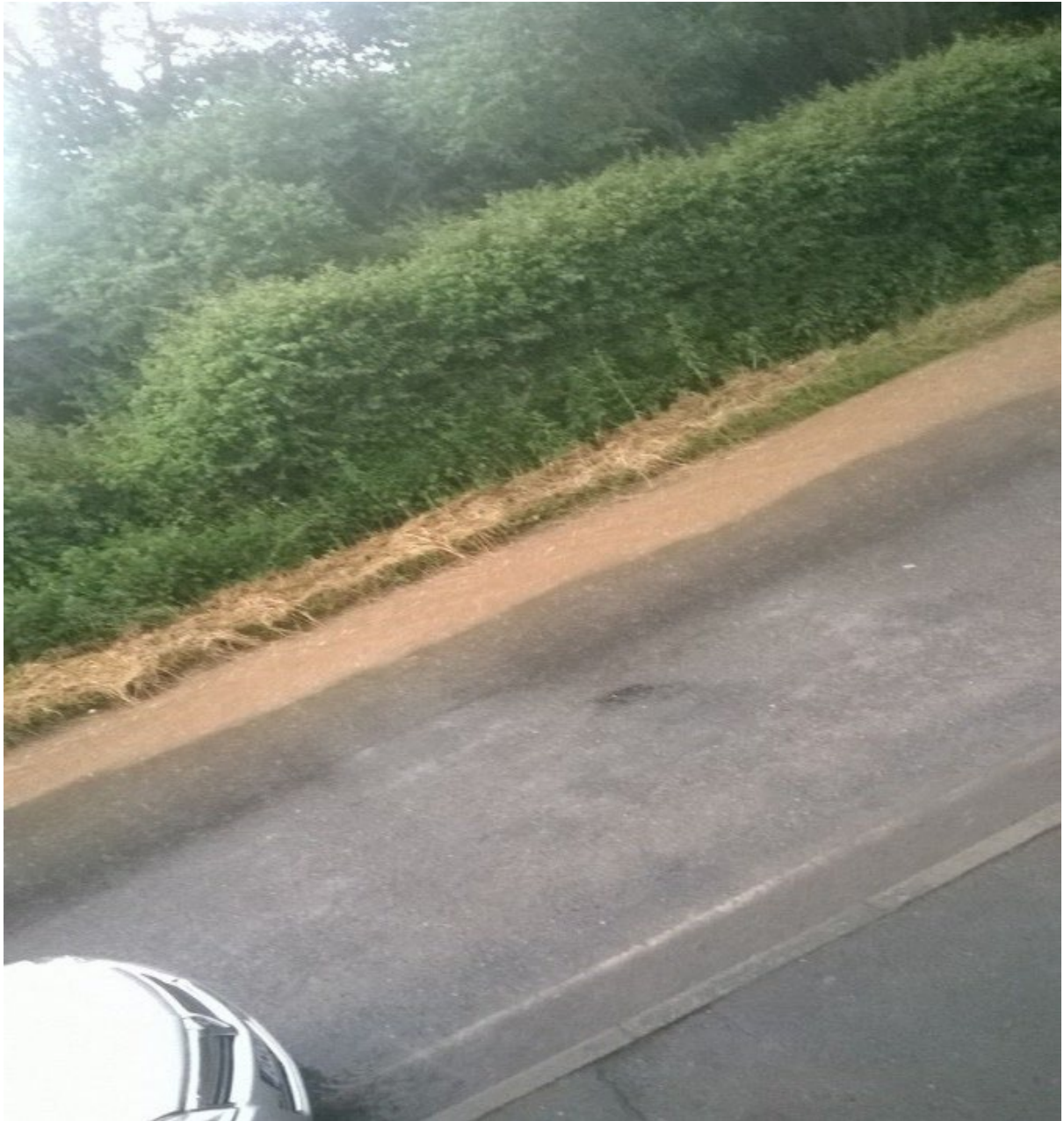
Breached ditch, Ickleton Road
