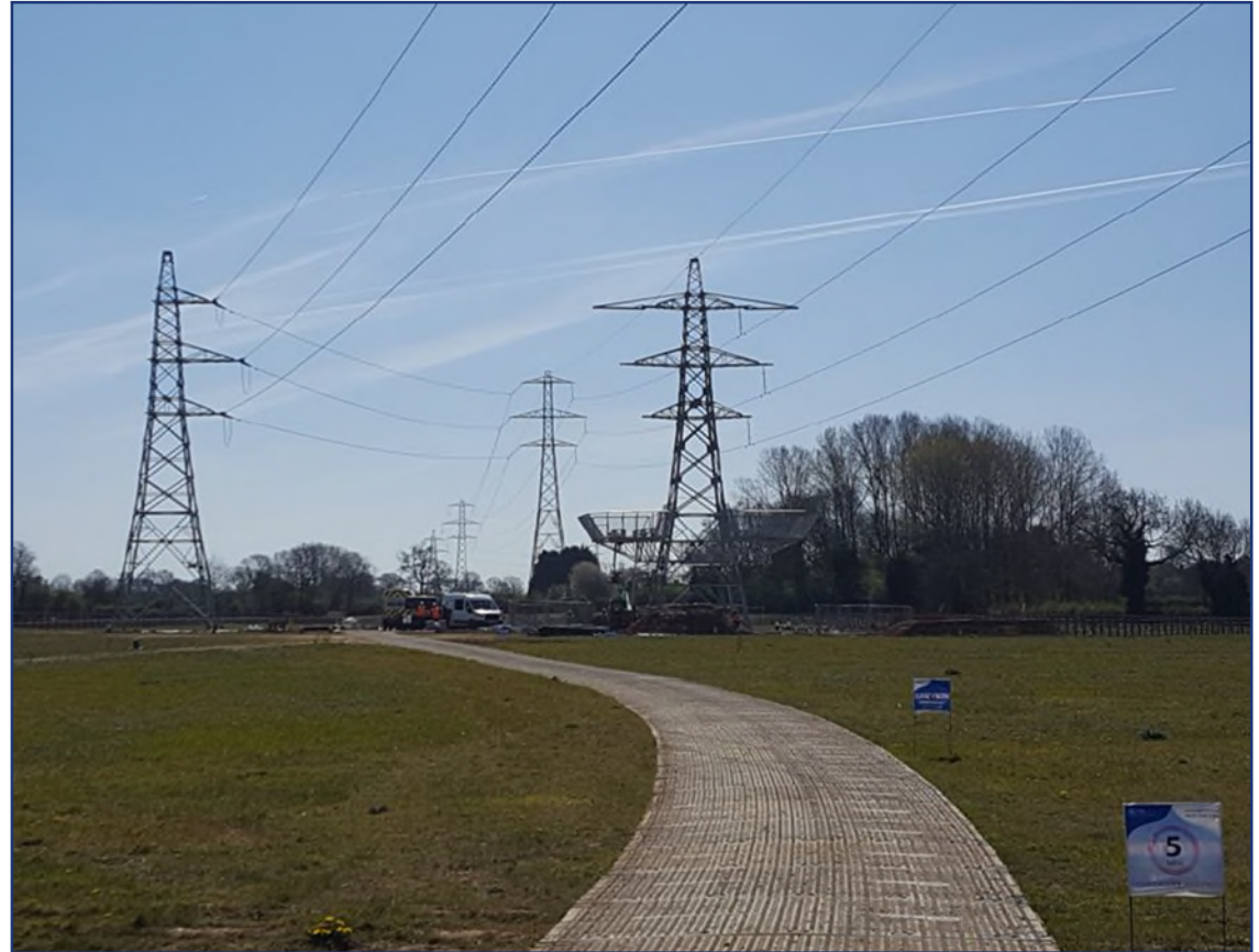
HS2 Phase One, National Grid Electricity Distribution Featherbed Lane site, near Brackley.
