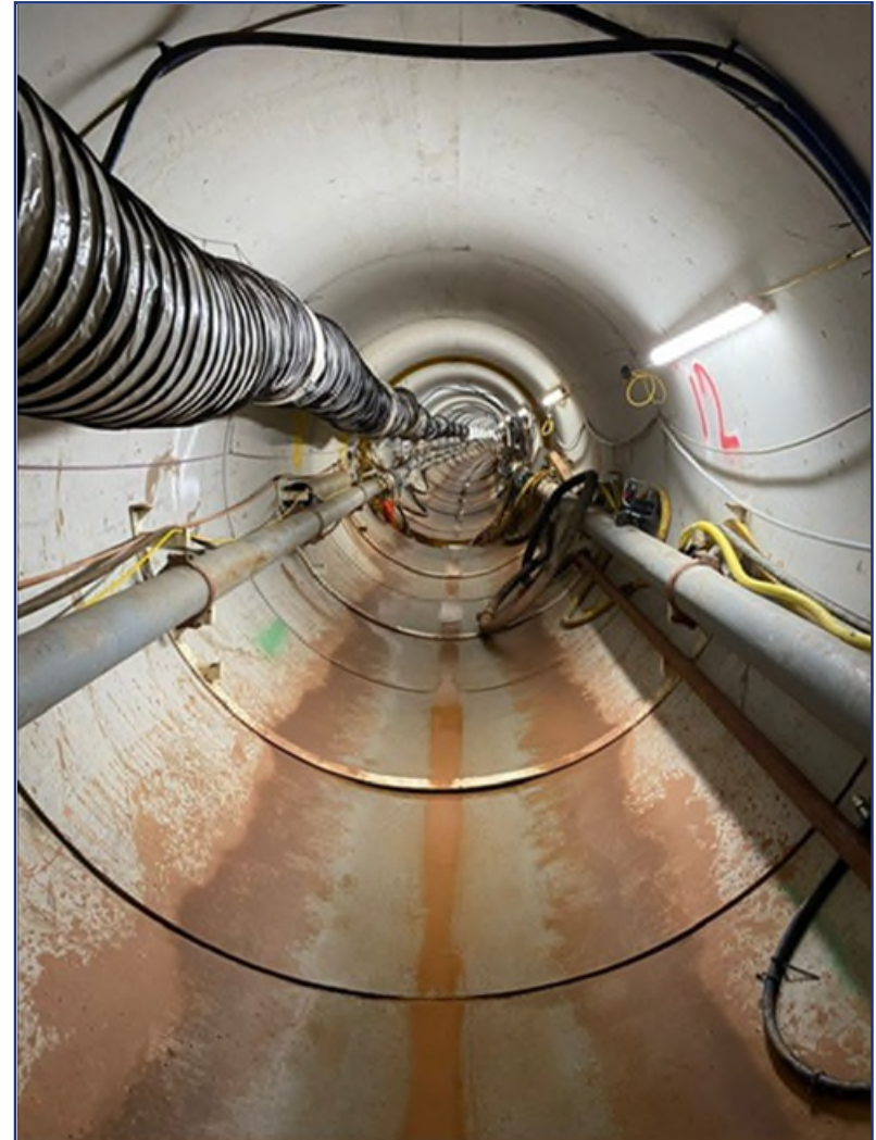
HS2 Phase One, 1800mm Sewer from the Erskine St Scheme in Birmingham under construction, with MTBM supply lines visible.
