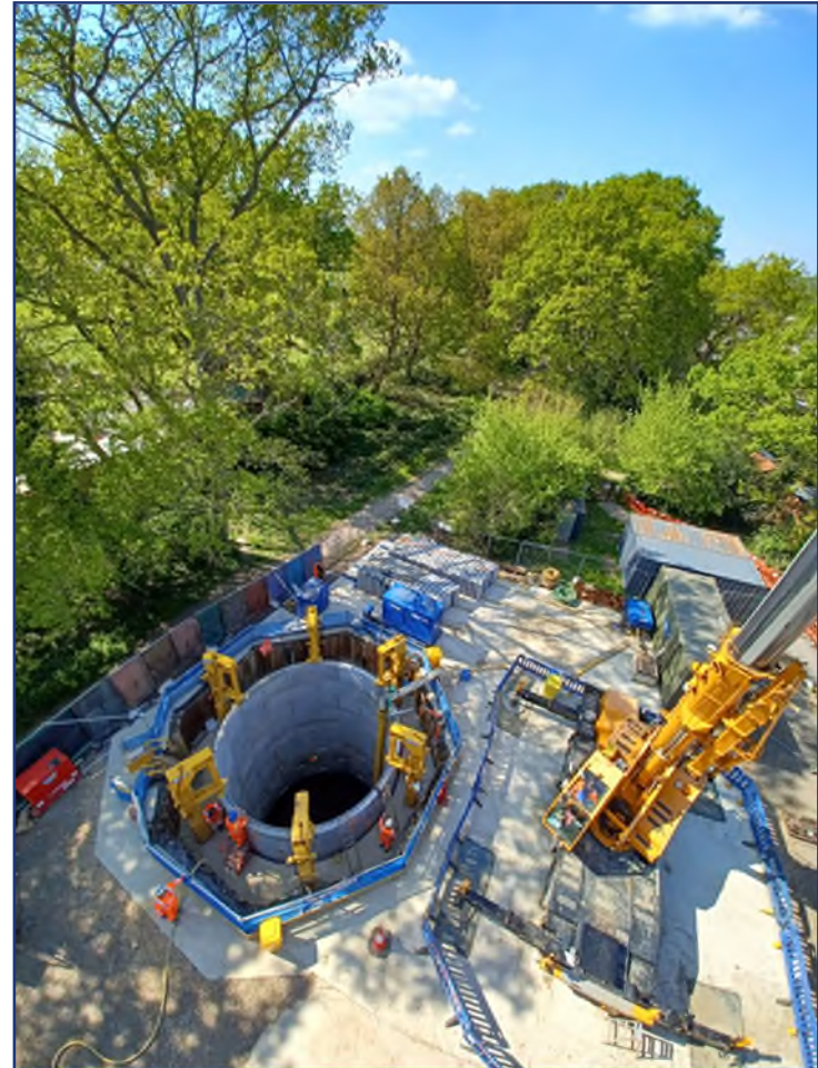
An access shaft for a TBM drive under construction at HS2 Phase 1 Thames Water Greenway site (West Ruislip), with precast rings jacked downwards, along with its dedicated crane and lifting platform.
