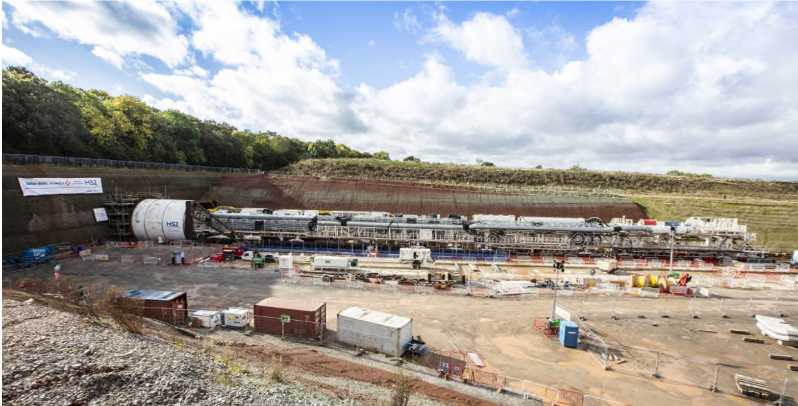
Bored Tunnel - HS2 TBM on site at Long Itchington Wood showing back up arrangements
