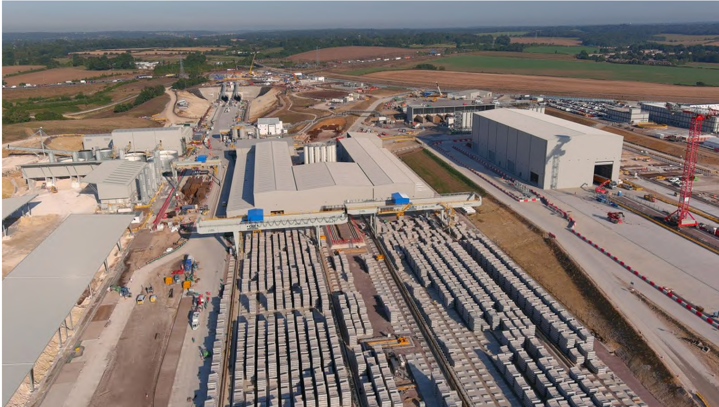
Bored Tunnel – Precast tunnel segments for tunnel ring construction at the South Portal site Chiltern Tunnel, Phase One
