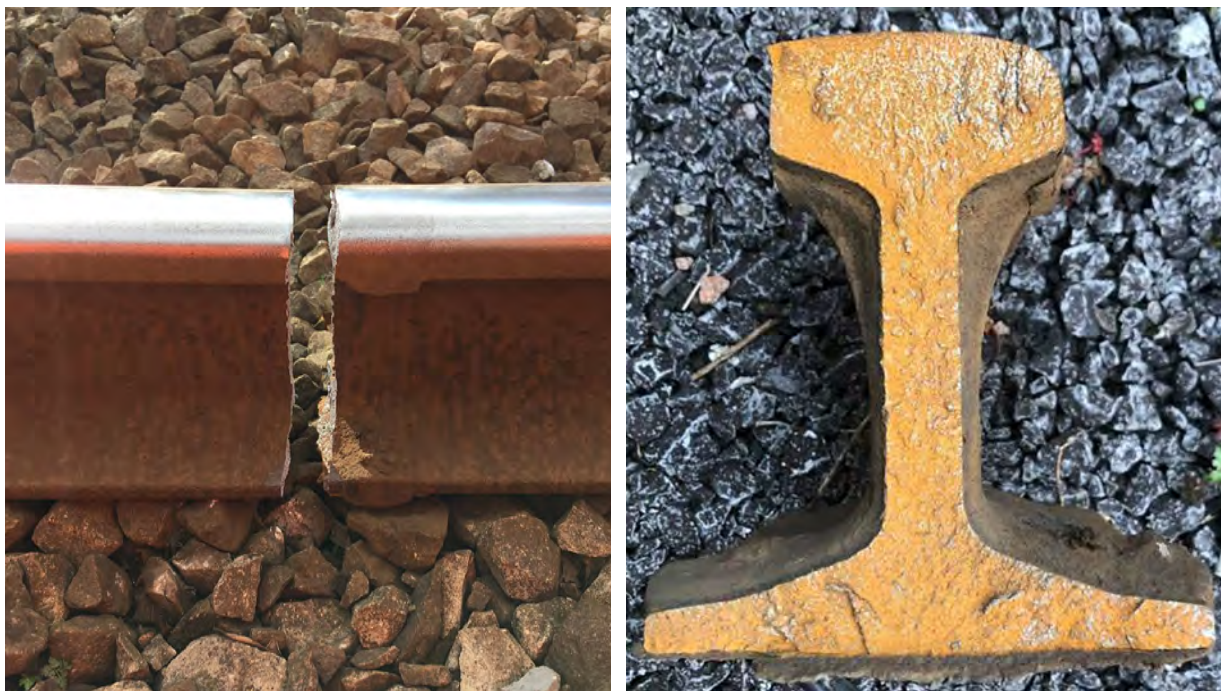
Figure 8: The rail break at Pencoed, in-situ (left-hand image) and its fracture face (right-hand image) (photos courtesy of Network Rail).
