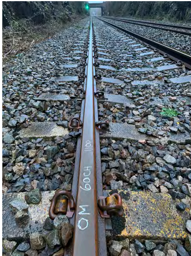
Figure 18: Railhead condition on the line between Lonlas Tunnel and Dynevor Junction (courtesy Network Rail).
