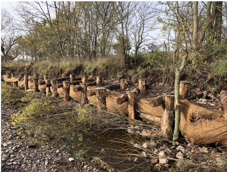
Figure 3: this picture shows a 'log matrix' technique used on the River Breamish where the section of bank was longer and higher.
