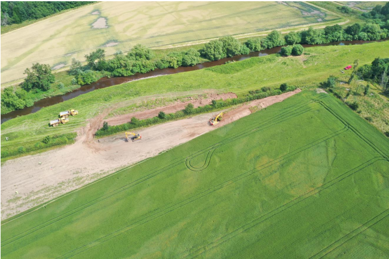
Figure 4: this picture shows the section of the River Glen where the existing flood bank is being set back.
