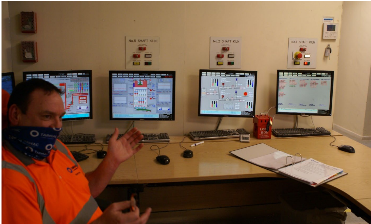
Figure 13: Control room showing SCADA user interfaces
