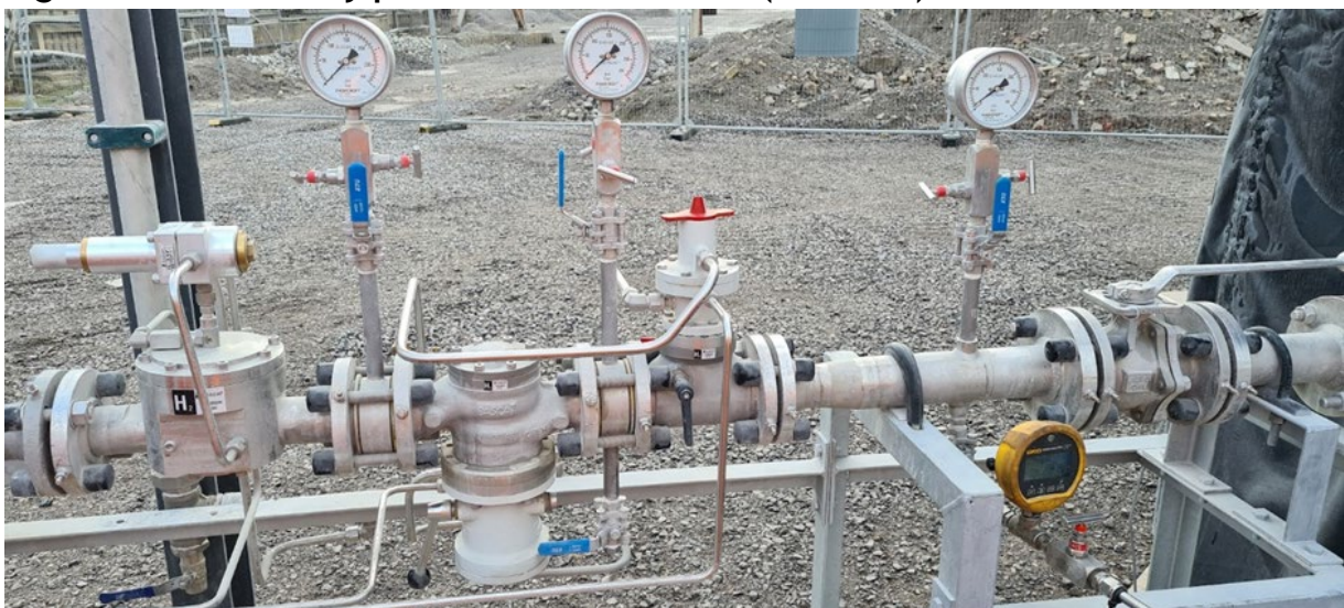
Figure 12: Secondary pressure let-down skid (FTP Skid)
